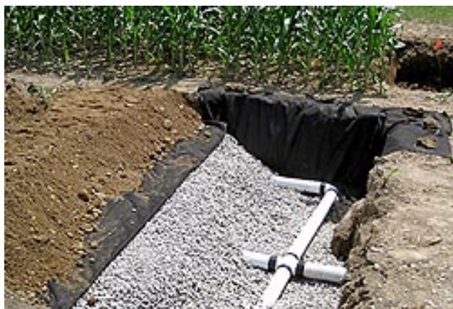
Image 9. Construction of a blind inlet. Septic tiles are placed on top of a layer of coarse limestone gravel, covered in a second layer of gravel, encased in landscape fabric, and backfilled with coarse soil to facilitate infiltration. (Credit: USDA).
