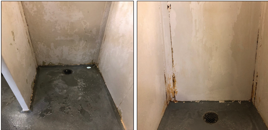
Figure 1. Poor condition of detainee showers as observed by DHS Office of Inspector General (OIG) on February 25, 2020.
