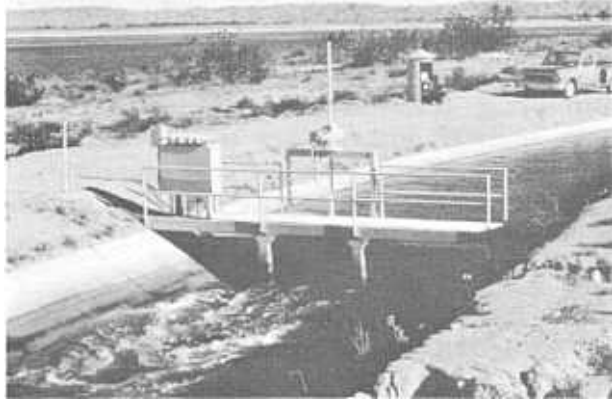
Prototype installation of automatic controls above a canal check. Photo P801-D-73319
