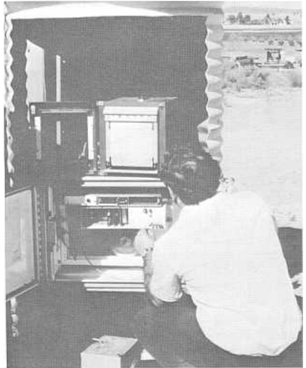
Closeup view of the EL-FLO Plus Reset Controller inside the stilling well just above the South Gila Canal Check No. 2. The electronic recorder above the controller and the Type F recorder below were used to collect data on equipment and canal performance. Photo P801-D-73318
