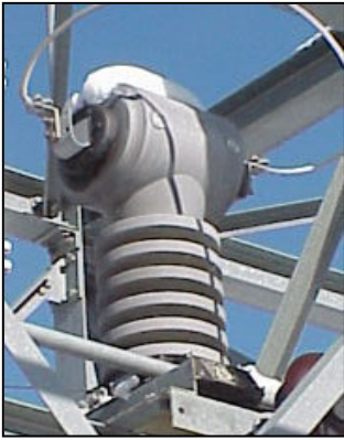
Current Transformer in Switchyard.
