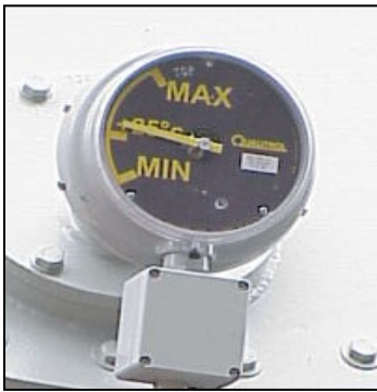
Figure 28 – Conservator Oil Level.
