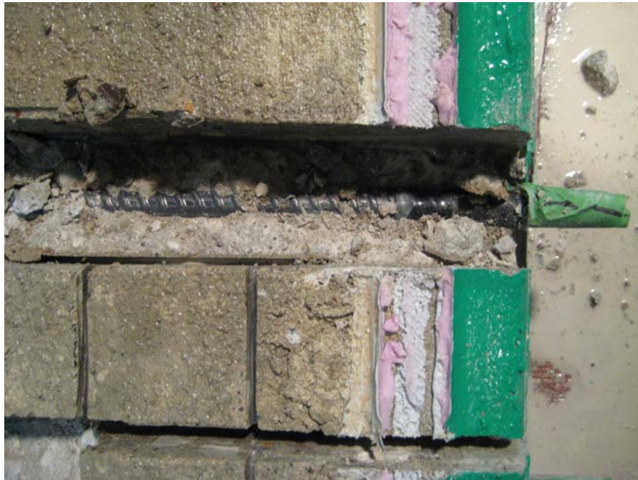
Figure 132 – Embedded rebar exposed without visible corrosion
