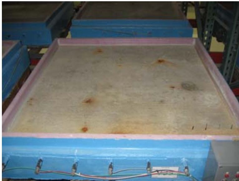
Figure 51 – Slab with cracked surface and small corrosion stained openings (0.75-inch cover, Batch #2, Slab 39)
