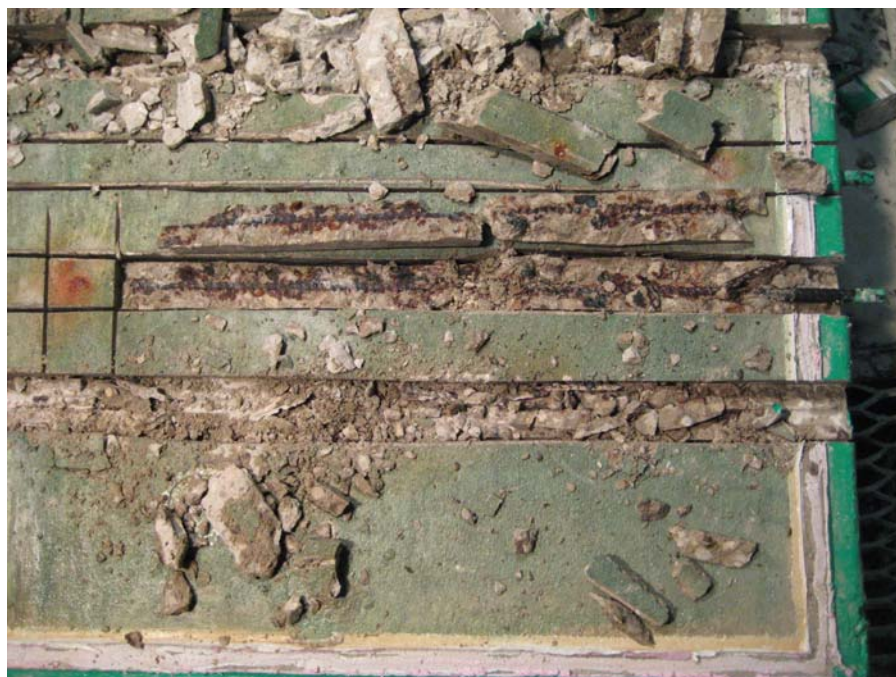
Figure 133 – Embedded rebar exposed with visible corrosion
