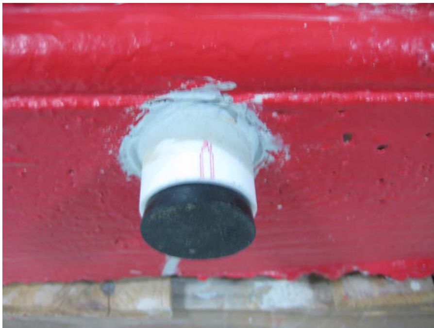
Figure 101 – Installed port for housing data-loggers
