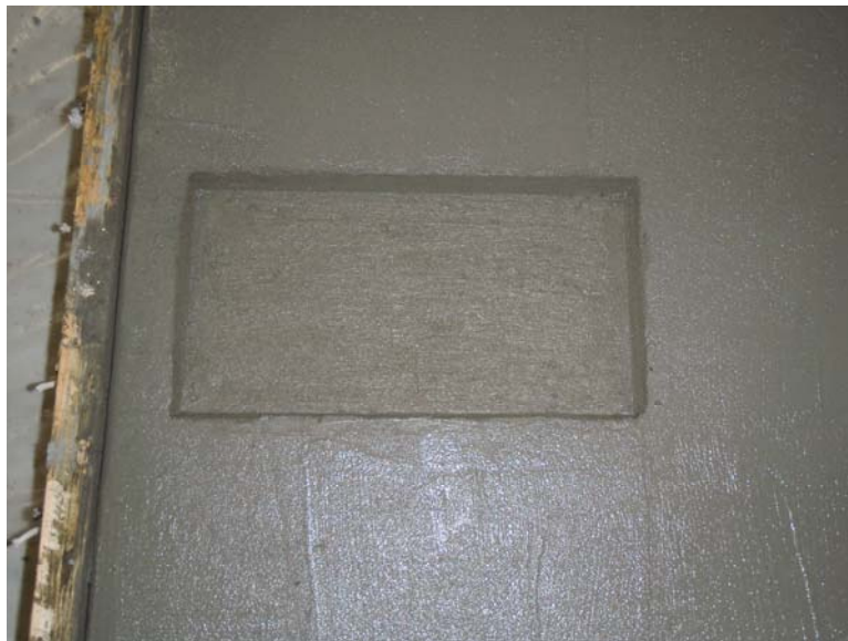
Figure 80 – Slab with depressed cover hotspot
