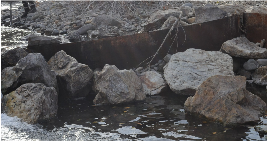
Figure 4.5 – Exposed metal support along structure cross bar (October 2008).
