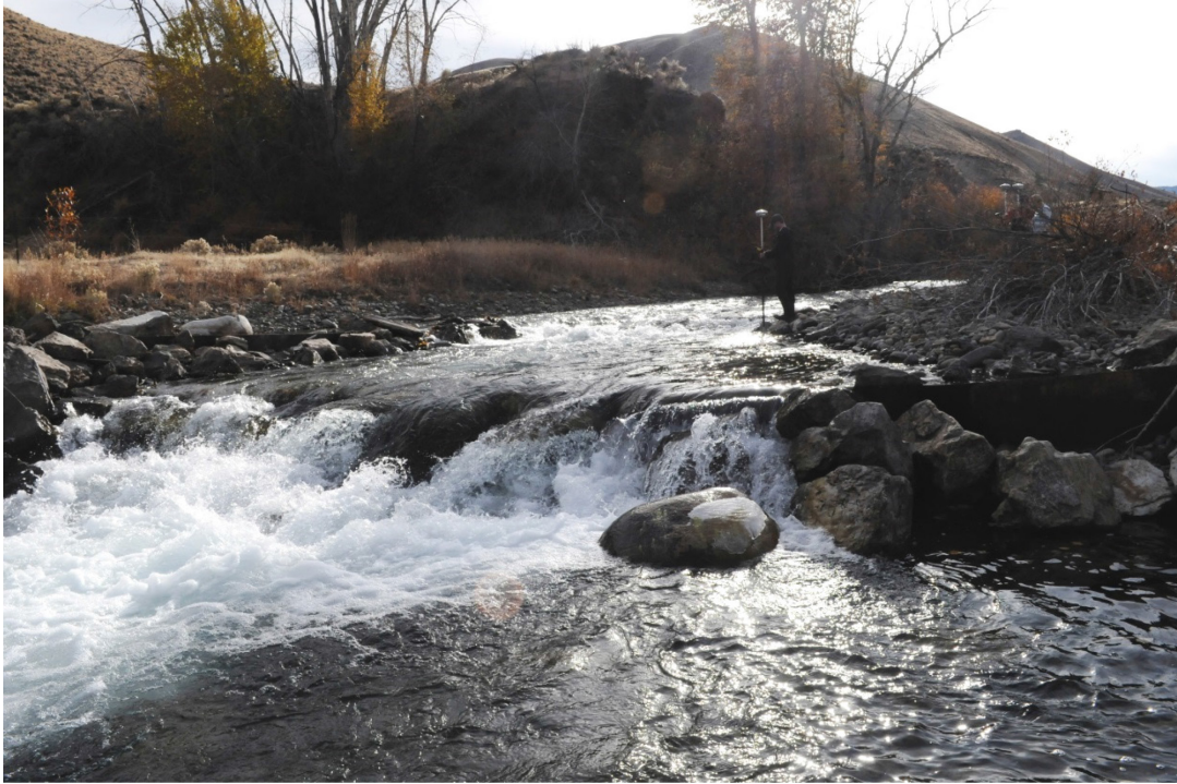
Figure 4.4 – October 2008. Note significant change in drop height since construction, mobilization of larger boulders, and excessive deposition upstream of structure.
