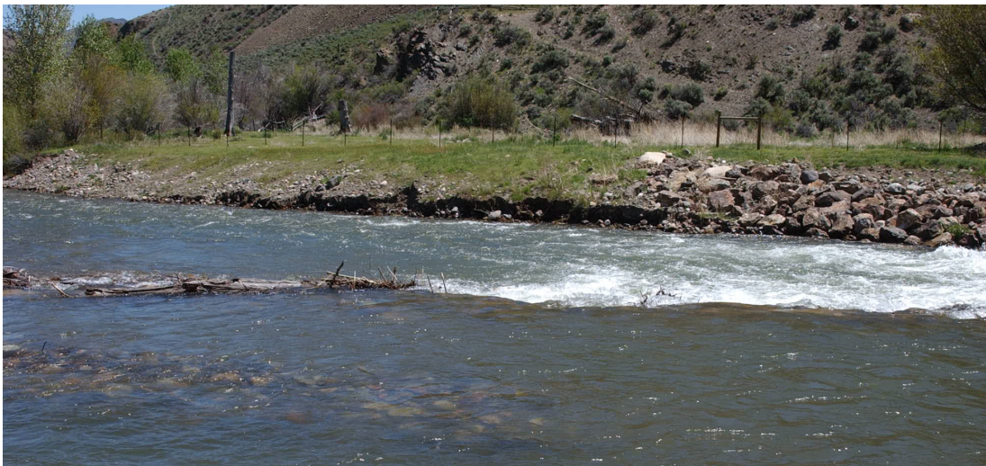
Figure 4.7 – Looking downstream of structure in May 2005. Note initial bank erosion along right bank.
