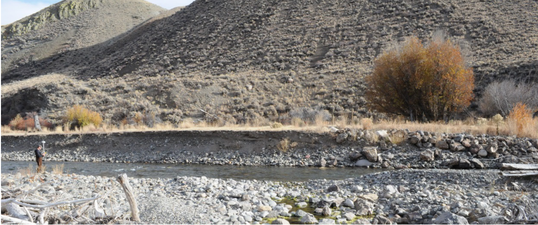
Figure 4.8 – Looking downstream of structure in October 2008. Bank erosion has resulted in destabilization of structure tie-in.
