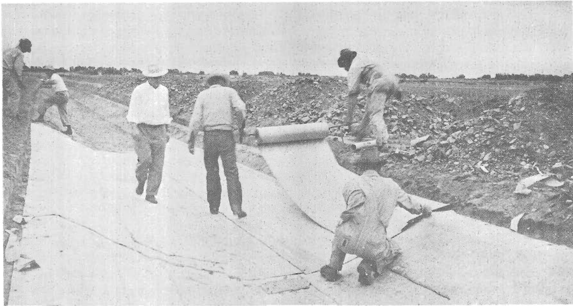
Figure 40.—Placing lightweight, buried, glass-fiber-reinforced, prefabricated asphalt canal lining on the Altus project, Oklahoma. CH-209-21.
