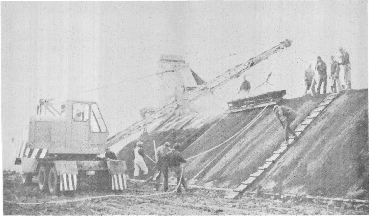
Figure 12.—Construction of 4-inch-thick asphaltic concrete lining on downhill side slope, New York Canal, Boise, Idaho. The lining is being joined to a vertical concrete cutoff wall near the toe of the slope. CH-538-60, November 1957.
