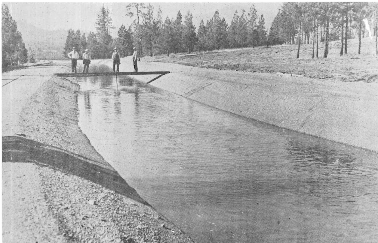
Figure 51.—View of completed canal lining with 6-inch layer of compacted earth and 6-inch protective gravel blanket shortly after construction in 1944. This installation is on the Rathdrum Prairie project, Idaho. 110-F-1484-C.
