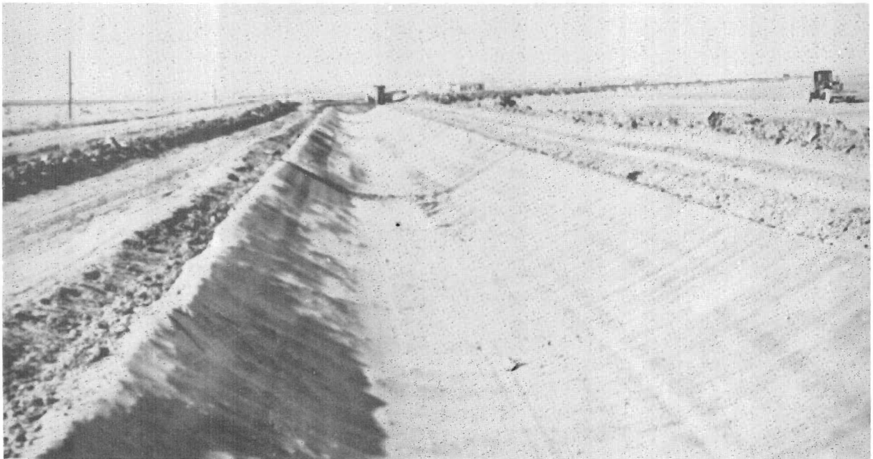
Figure 47.—Approximately 1,000 feet of 1/32-inch-thick butyl lining in place and ready for cover in the Bugg Lateral, Tucumcari project, New Mexico. P257-D-25961.
