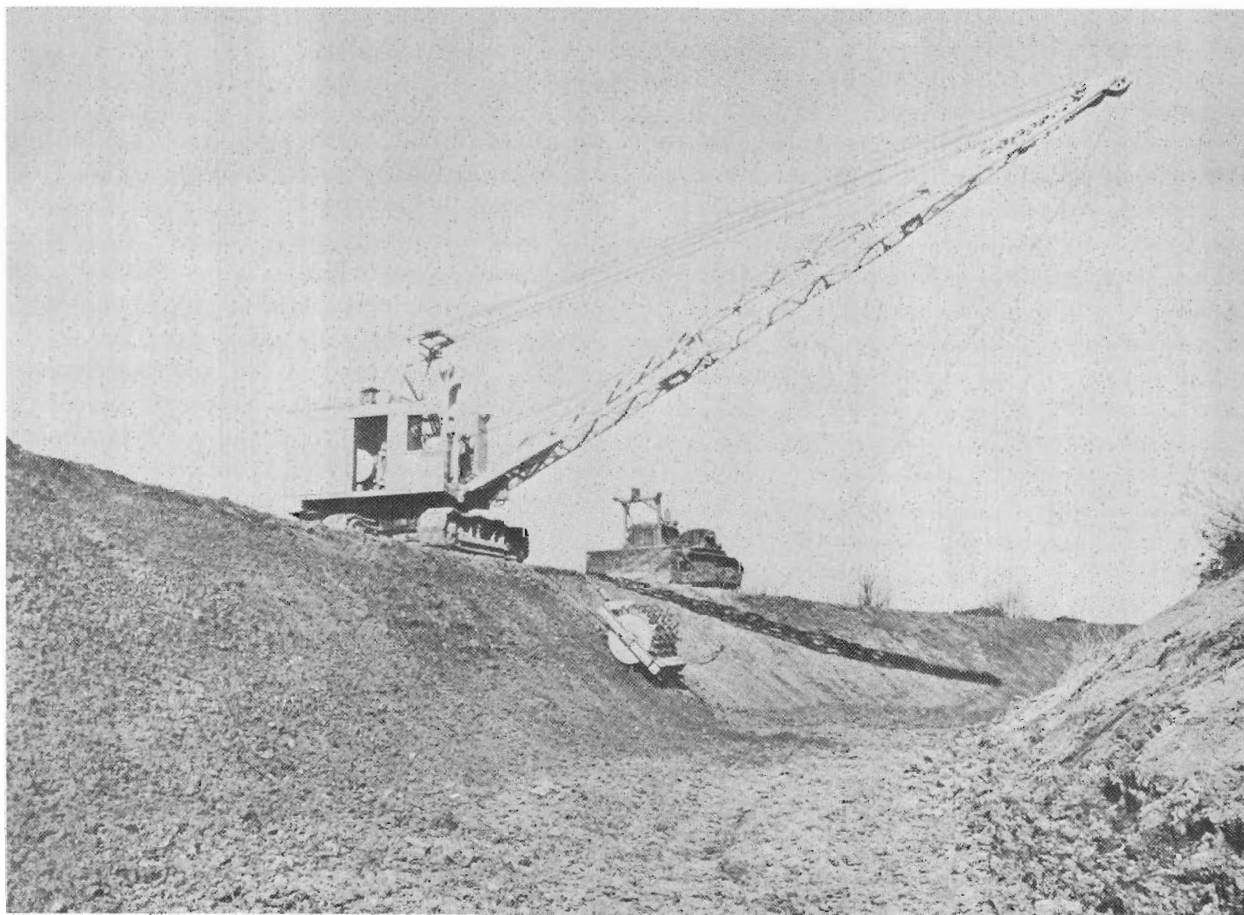
Figure 50.—Transverse compaction of thin earth lining (two 6-inch layers) by use of a single-drum sheepsfoot roller on the W. C. Austin project, Oklahoma. PX-D-32052.
