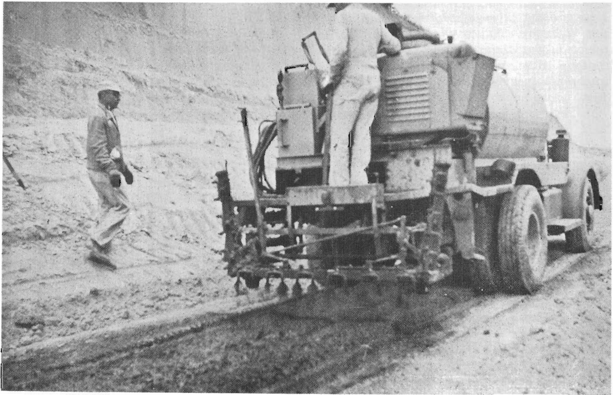
Figure 55.—Applying asphalt emulsion to soil with 1,000-gallon-capacity asphalt distributor, for soil stabilization. CH-575-1.
