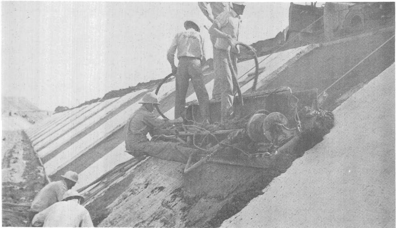
Figure 23.—Lining a portion of the Courtland Canal, Missouri River Basin project, Kansas, by use of a winch-drawn screed operating transversely up each side slope. P271-701-1641.
