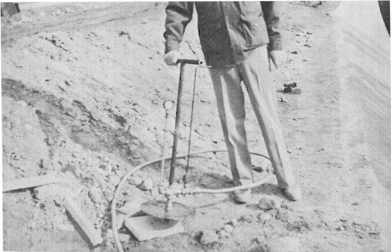
Figure 60.—Closeup view of an asphalt undersealing gun which was fabricated from standard pipe and fittings. PX-D-14667.
