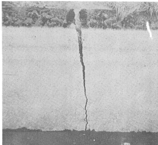
Figure 10.—Typical cracks caused by low temperature ( -30^{\circ} F.) in a 2-inch-thick asphaltic concrete canal lining in the State of Washington. P222-D-15355.
