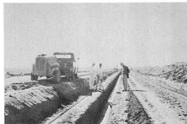
Figure 67.—An inflated tube of balloon cloth serving as an interior form for cast-in-place, reinforced, monolithic, concrete pipe. P25-D-15286 and P25-D-15284.
