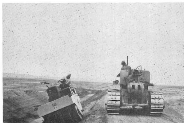
Figure 33. —Compaction of soil-cement on lateral side slopes with a self-propelled pneumatic-tired roller attached by cables to a tractor for support. PX-D-32562.
