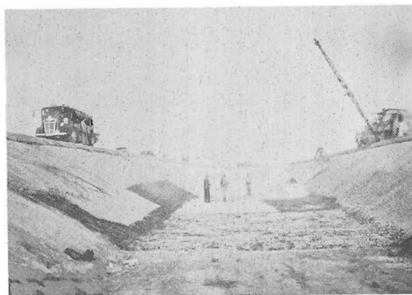
Figure 14.—Construction of penetrated macadam, showing application of catalytically blown asphalt cement at 400° F., on the Madera Canal, Central Valley project, California. PX-D-32054.
