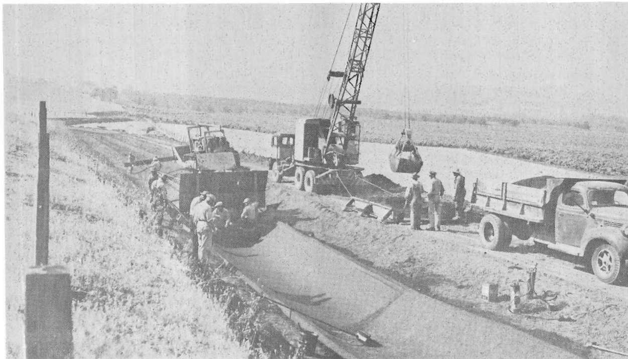
Figure 11.—Hot asphaltic concrete lining being applied to canal prism by tractor-drawn slip-form. CH-102-26.
