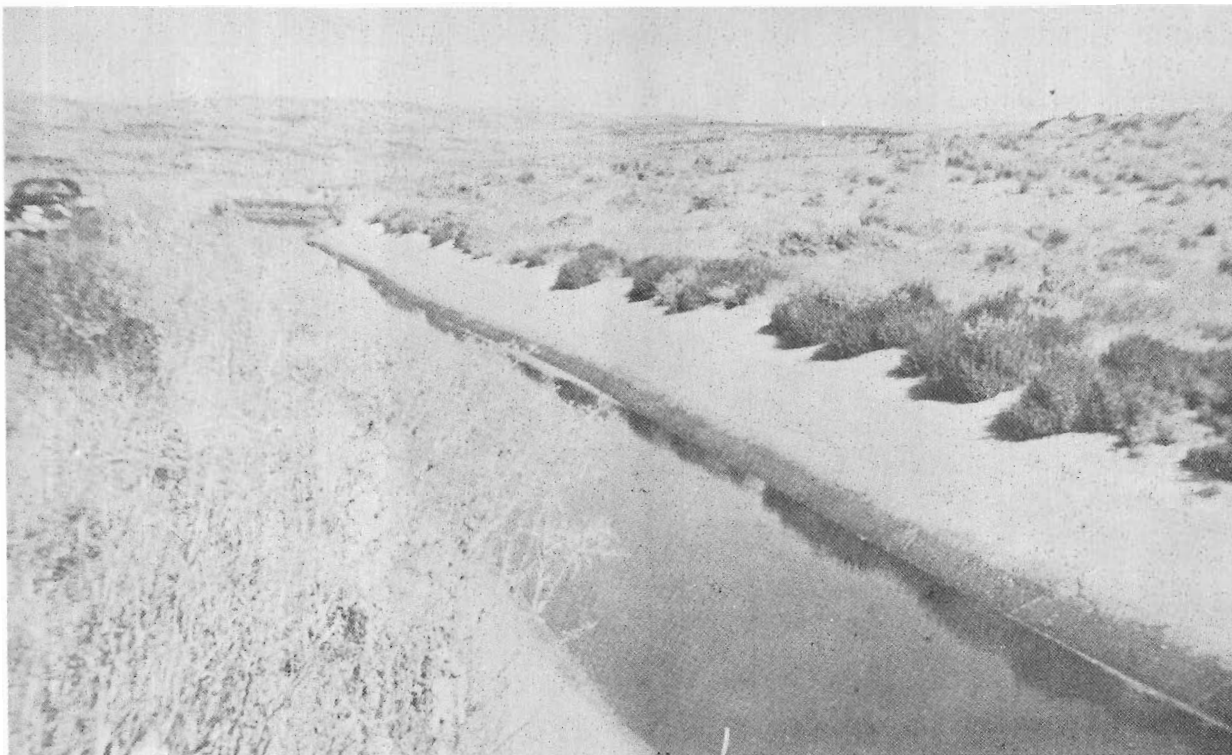
Figure 32. —A plastic type soil-cement lining placed on the Boise project in 1948 which is still in good condition after 14 years of service. Although the lining shows some evidence of scaling, a few local eroded pockets, and some cracking, it is still serviceable and effective in controlling seepage losses. P3-D-15424.
