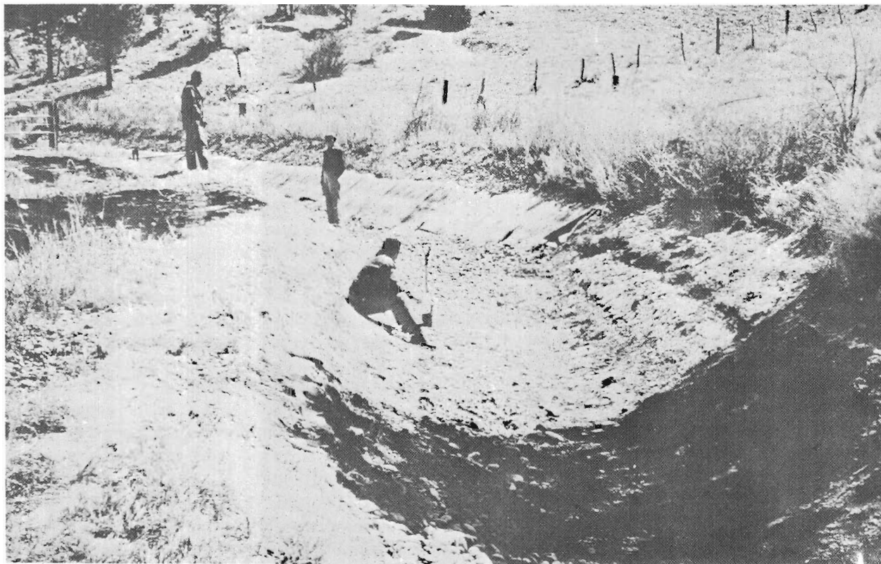
Figure 30.—A plastic material which has failed in three reaches where placed as an exposed membrane, due to weathering and erosion. The only remnant of the exposed plastic is that along the top of the canal side slopes. Lining in the background is an exposed type prefabricated asphaltic material. P11-D-14991.
