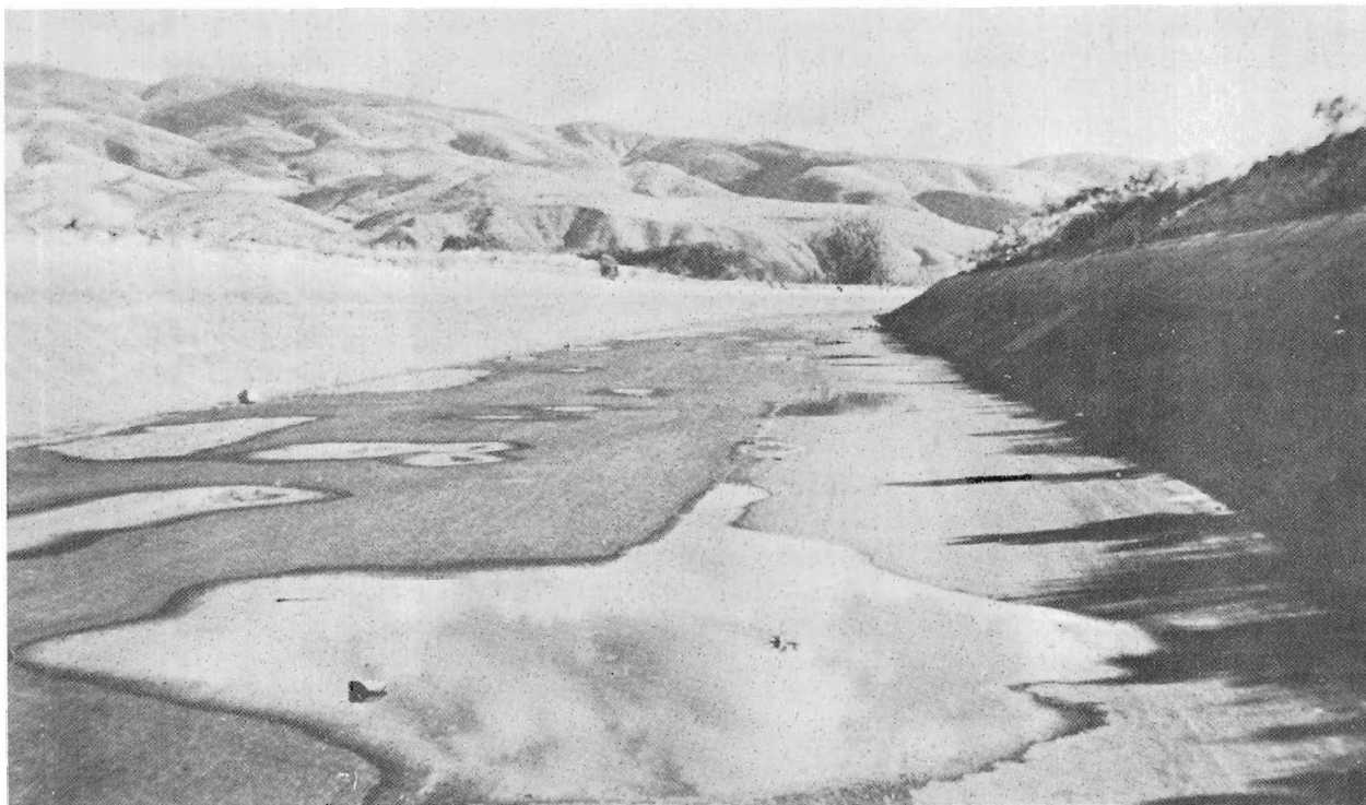
Figure 25.—Bottom of the Main Canal, Boise project, Idaho, 14 years after resurfacing with hot-plant-mixed asphaltic concrete. Examination disclosed no cracks or signs of failure in the entire length. The resurfacing was placed in 1944 to repair a deteriorated portland cement concrete lining. P3-D-15373.
