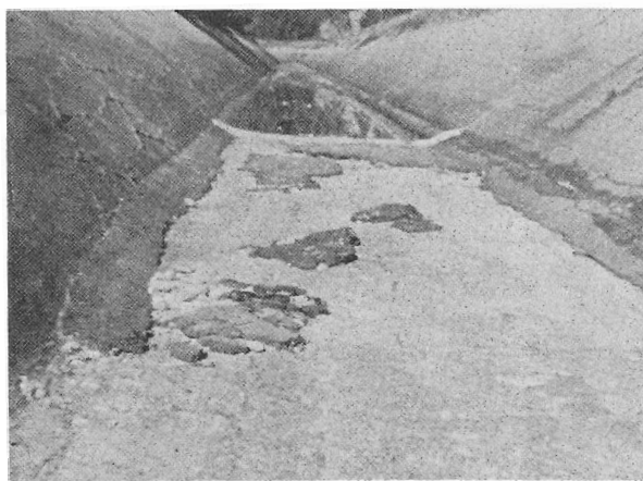
Figure 26.—Asphaltic concrete resurfacing that has failed at the lower end of the lined reach due to poor bond to underlying concrete and uplift pressure. The condition of the deteriorated portland cement concrete is shown in the immediate foreground. P-33-D-15360.
