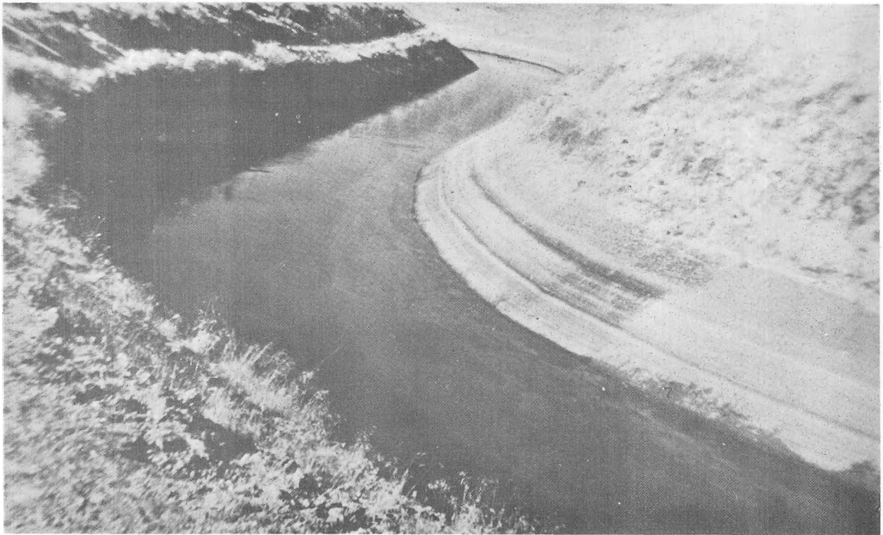
Figure 9.—A hot-mixed, asphaltic concrete canal lining after being in use for 15 years in the northwestern United States. P3-D-15353.
