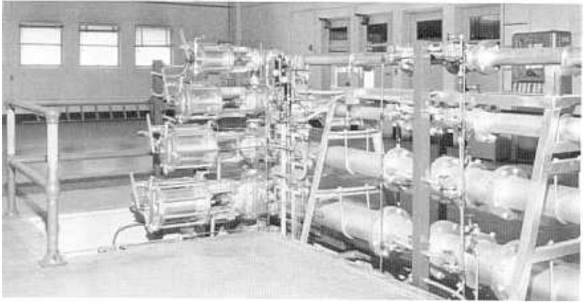
Figure 1-5.—Venturi meters and hydraulically controlled throttling valves in pump discharge lines. P801-D-79237
