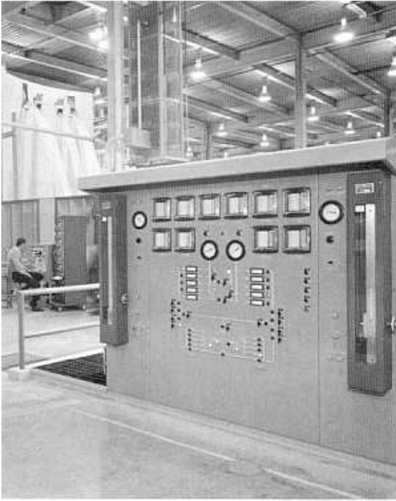
Figure 1-4.—Control board. P801-D-79238
