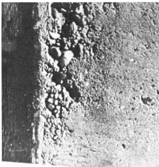
B. Erosion of concrete resulting from cavitation caused by a 6-millimeter offset between steel gate frame and concrete guide wall.
