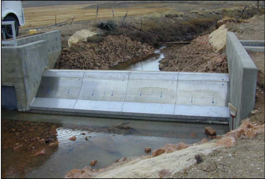
Figure 5. Coanda screen at Lake John near Walden, Colorado.
