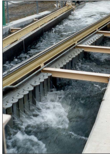
Figure 31. Adjustable baffles located behind fish screen panels.
