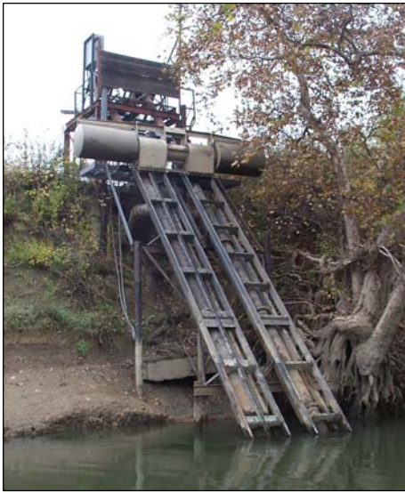
Figure 7. Retractable submerged cylindrical screen on Sacramento River near Grimes, California.
