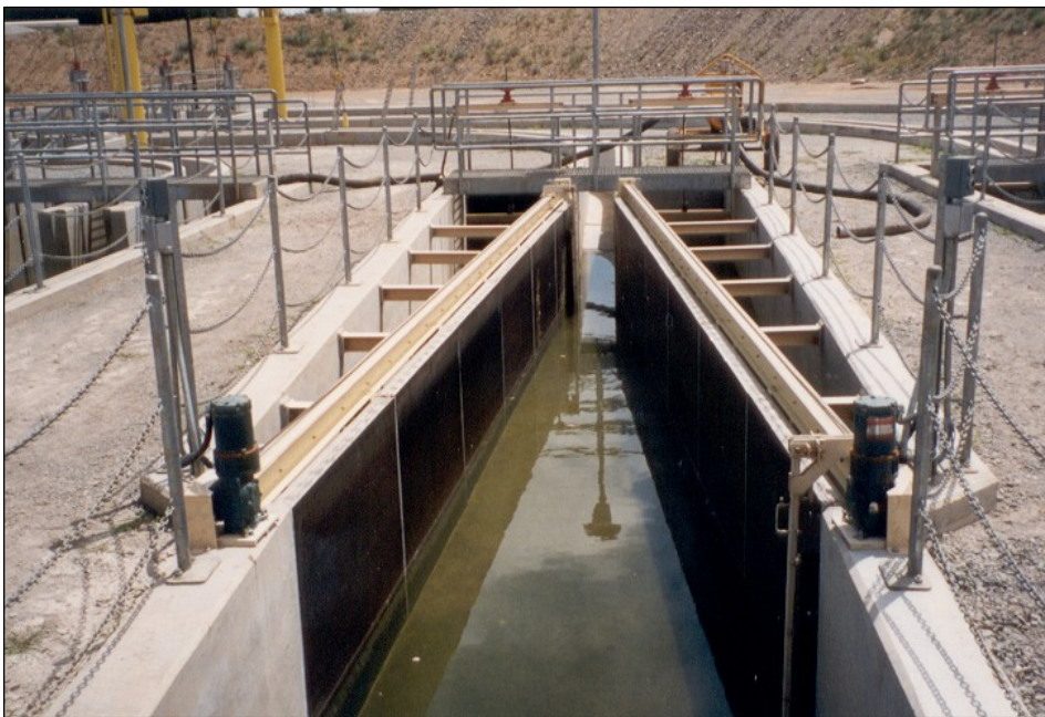
Figure 30. Flat plate V-screen with a terminal fish bypass.
