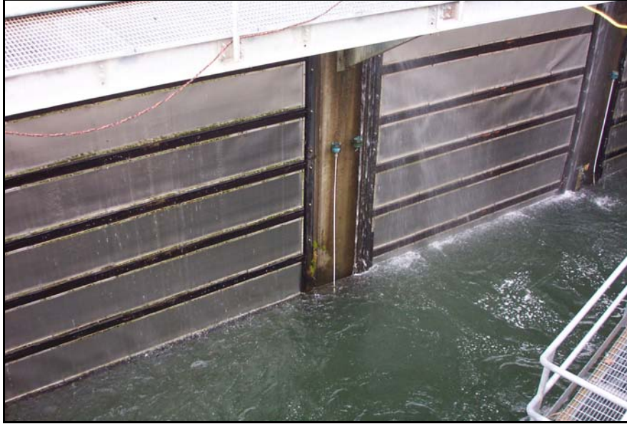
Figure 3. Multiple traveling screens at Roza Fish Screens Facility near Yakima, Washington.
