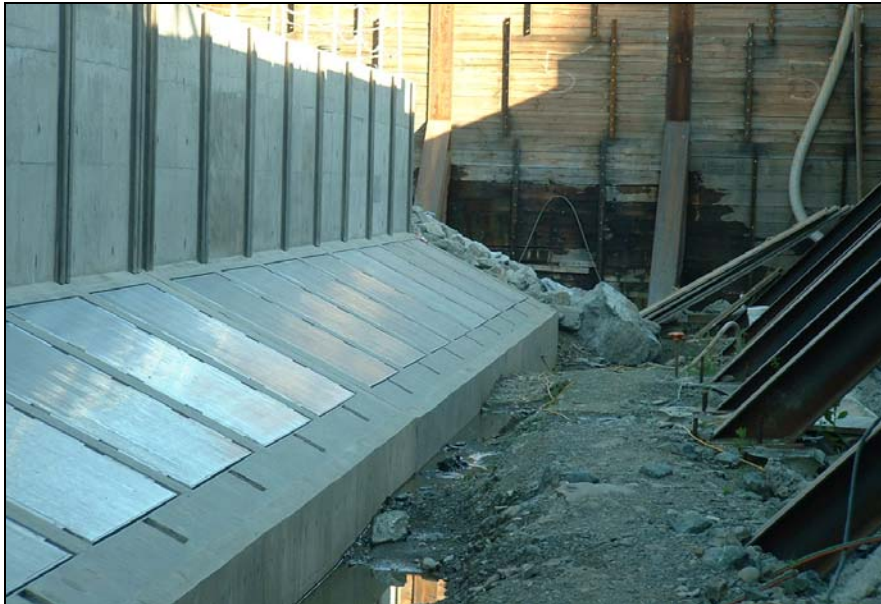
Figure 4. Inclined screens at Savage Rapids Diversion near Grants Pass, Oregon.
