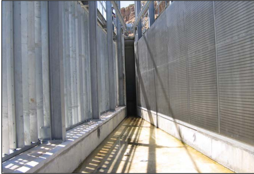
Figure 1. Government Highline Canal in-canal V-screen near Grand Junction, Colorado. This construction photo shows the wedge-wire flat plate screen panels (right), vertical baffles (left), and fish bypass intake (center).
