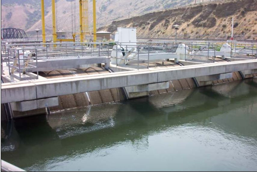
Figure 26. Rotating drum screens in one bay of Roza Fish Screens Facility.
