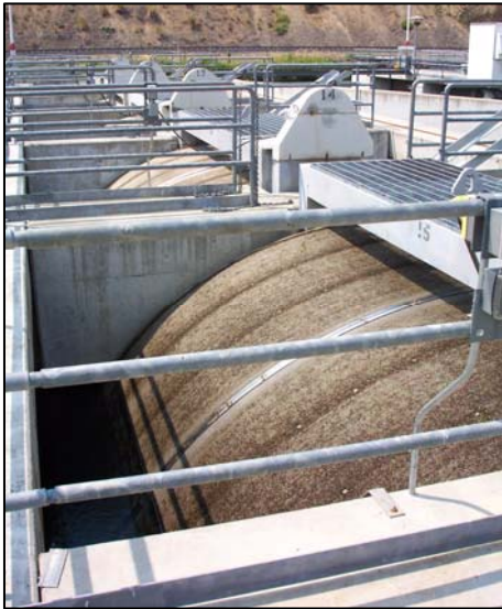
Figure 6. Rotating drum screens at Roza Fish Screens Facility near Yakima, Washington.
