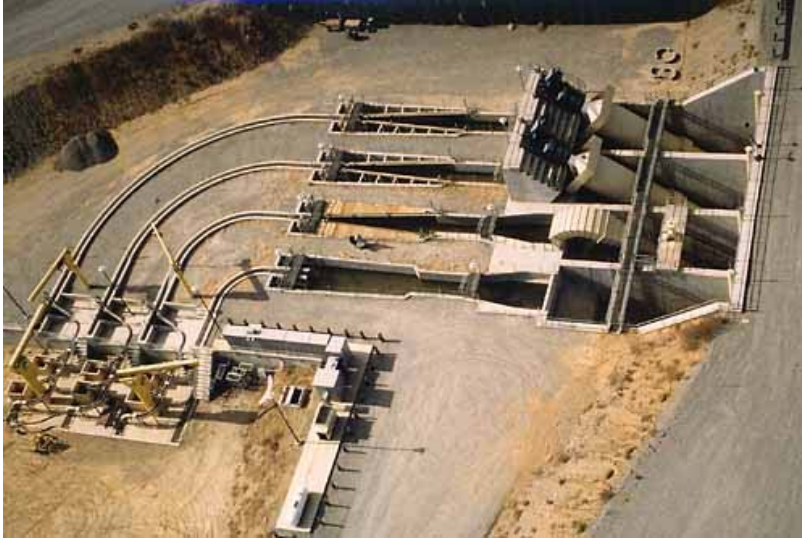
Figure 29. Overview of Red Bluff Research Pumping Plant.
