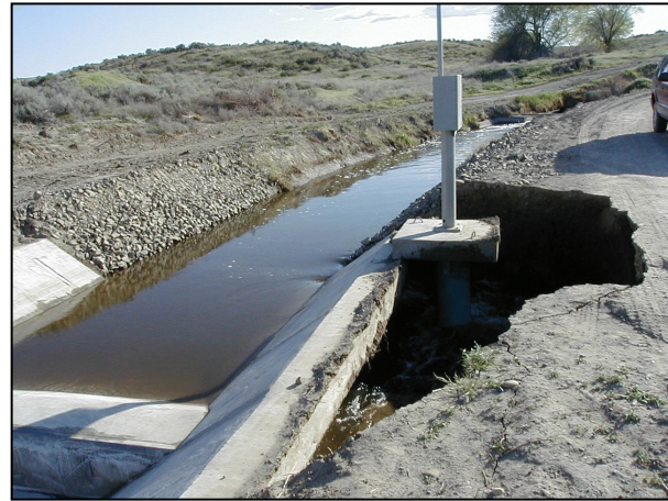
Figure 63. —A canal drop structure that failed by side seepage.
