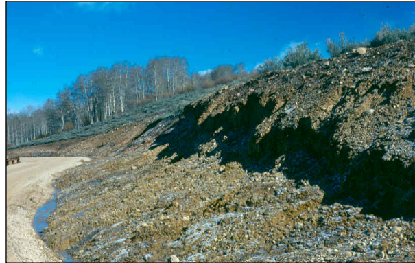
Figure 58. —A slide occurred where moisture entered a low density material.
