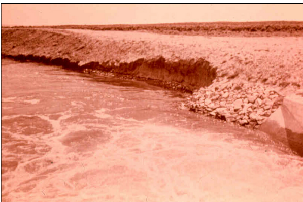
Figure 57. —Undercut erosion due to water flow.
