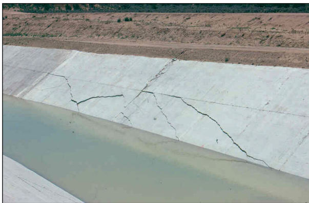
Figure 70. —Canal lining cracking due to frost heave.
