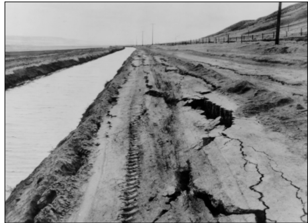
Figure 48. —Cracking and settling of canal bank in dry, low density silt [1].
