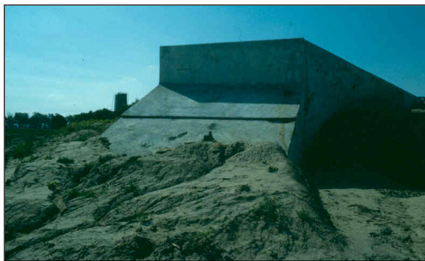
Figure 65. —This structure was placed on uncompact material, causing differential settlement of the structure.
