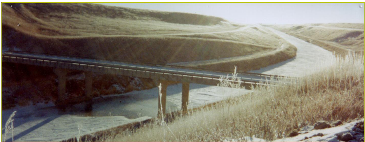
Figure 61. —The slide was fixed by cutting back the slopes and reducing the waste pile and spreading it over a larger area. Horizontal drains were drilled both above and below the lower O&M road.
