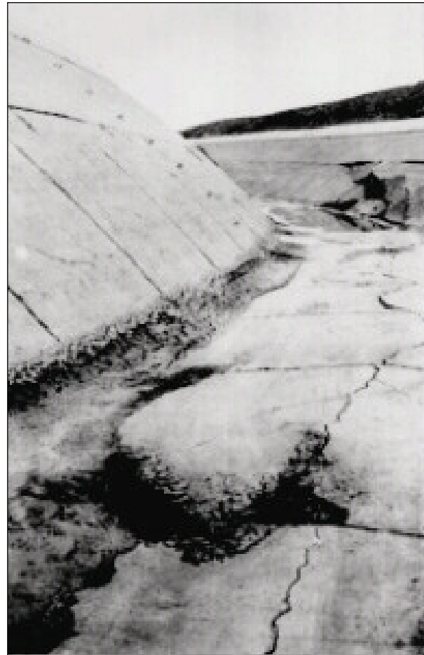
Figure 53. —Soil expanding below a canal lining.
