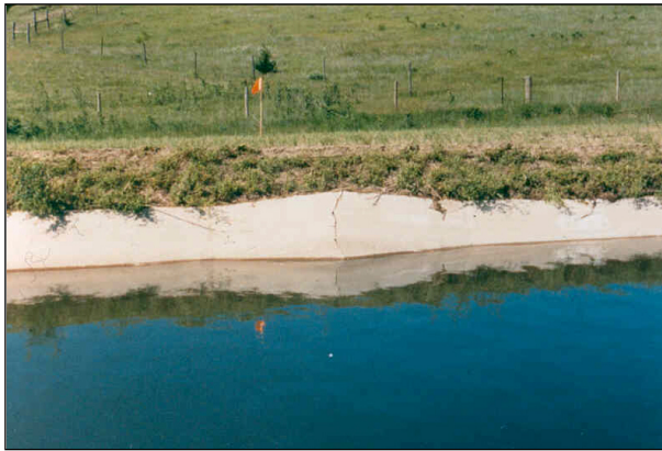
Figure 69. —Frost heave of a canal lining with drainage toward the canal.
