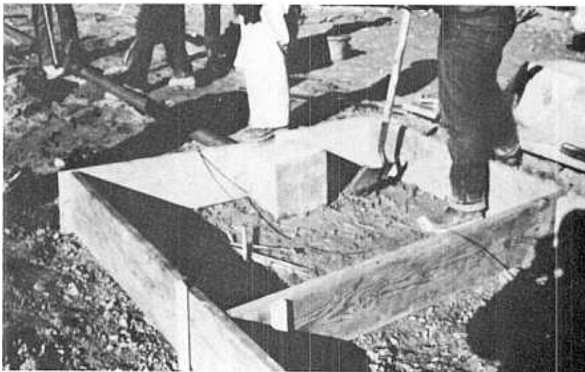
Figure 4-29.—Far end of radiosonde installation. P801-D-81024.
