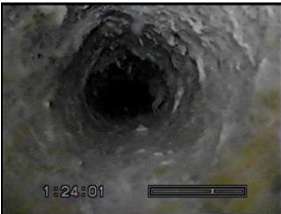
Figure 49. — Bacterial growth is shown completely covering the 8-inch diameter HDPE pipe.
