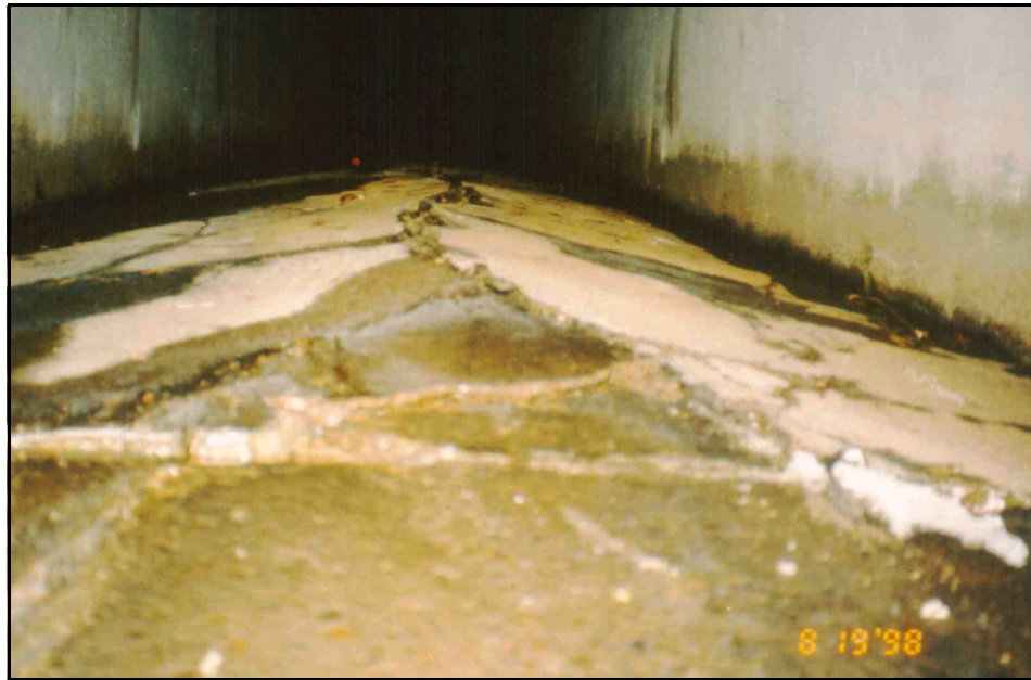
Figure 29. —Grassy Lake Dam Spillway, Wyoming—Chute floor has succumbed to inadequate drainage provisions and frost heave.
