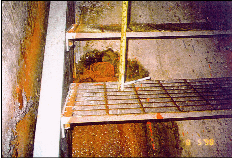
Figure 7. —Red clay oozing from a drain under a sloping staircase. The plumber's packer that had capped the hole was pushed out by the pressurized mud.
