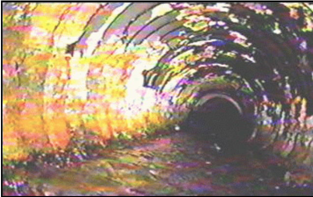
Figure 102. — Extensive deterioration existing within a CMP pipe.
