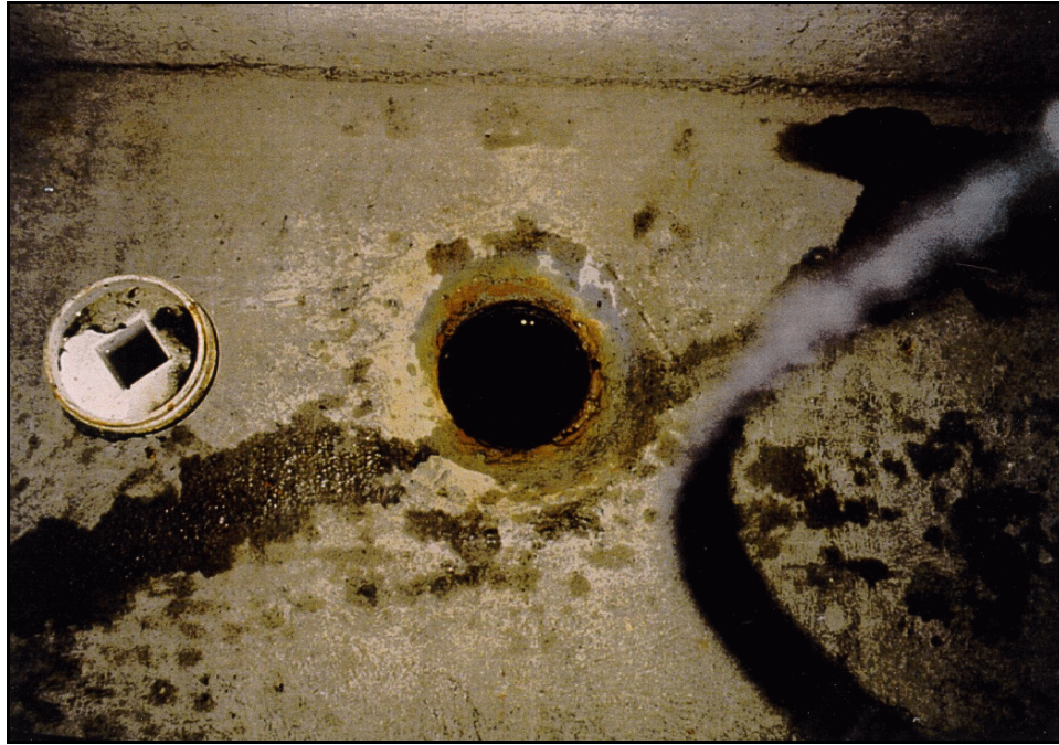
Figure 13.—Top of a drain hole with a 4-inch threaded cap. The pipe is 4 inches in diameter, and the hole becomes 3 inches upon entering bedrock.
