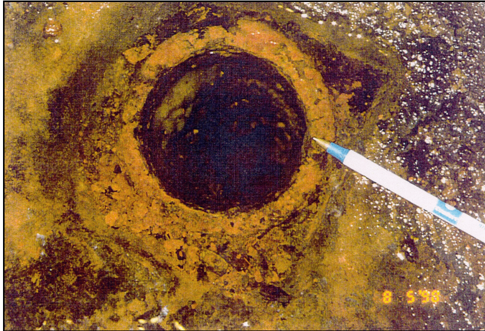
Figure 5. —Top of a drain showing the rusted out threads in the 3-inch steel pipe and the deposit of iron bacteria in the upper part of the hole.
