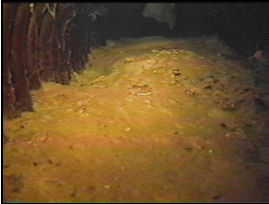
Figure 89. —The typical amount of sediment deposition observed in toe drain pipes in a November 2000 inspection.
