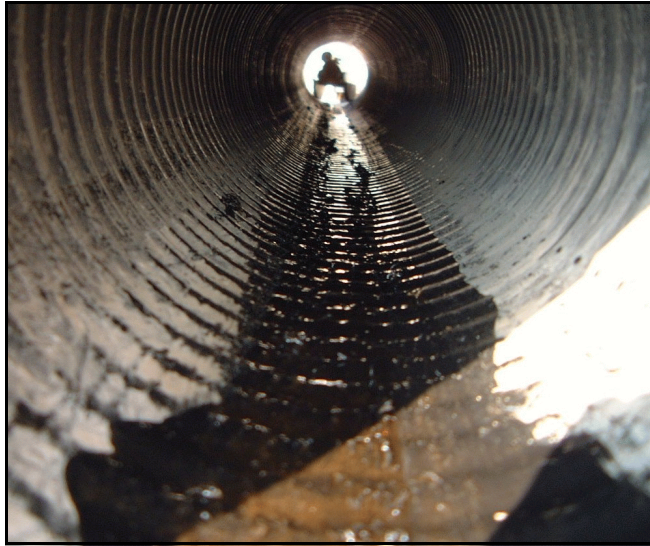
Figure 25. —Example of the slippery invert condition.
