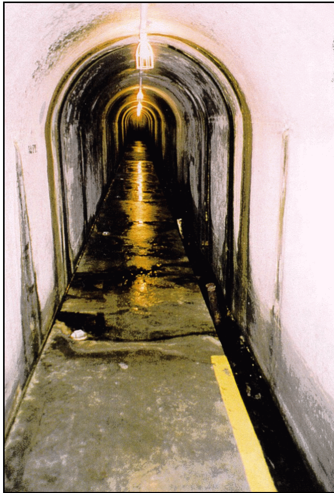
Figure 12. —Drainage ditch located along the upstream side of the access tunnel or gallery. Water is passed from the drain holes into the drainage ditch through a 2-inch steel pipe embedded in the concrete floor. This view looks along the right abutment foundation drainage tunnel.
