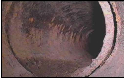
Figure 104. —Concrete pipe experiencing extensive joint offset and separation at a bend in the pipe.
