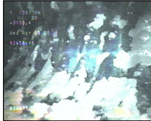
Figure 103. —CMP pipe experiencing extensive loss of surface coating due to delamination.
