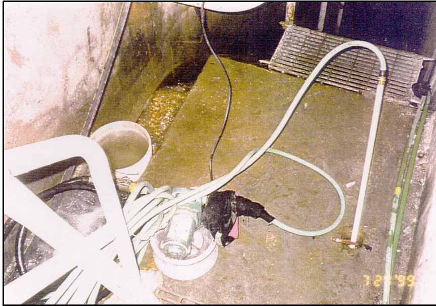
Figure 38. —Electric pump, garden hose, and flush-jointed PVC used to flush drains before making an initial down-hole video examination. Water was obtained by placing a temporary dam in the nearby drainage gutter.
