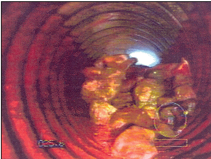
Figure 93.—CMP outfall pipe with coarse grained material.
