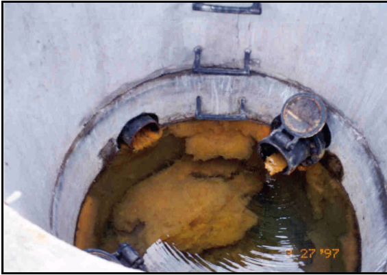
Figure 42. —The manhole shows an example of biofouling
