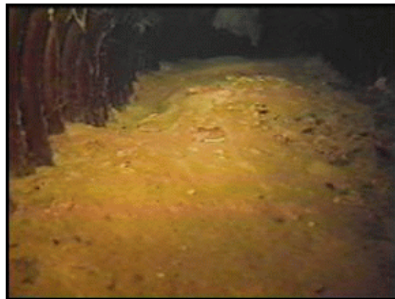
Figure 52. —Sediments were observed fouling the invert portion of a 12-inch diameter HDPE pipe.
