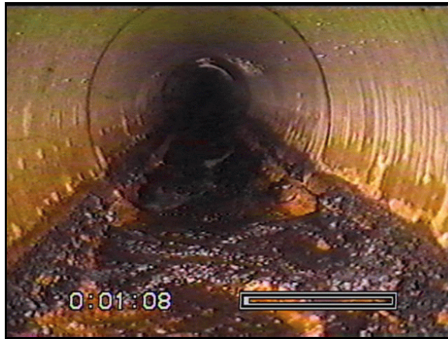
Figure 23. —Example of bacterial growth encountered during a video inspection of a toe drain.
