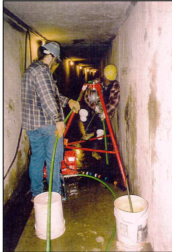
Figure 31. —Green flexible lance hose being lowered into a drain using the tripod with electric winch that is being used to help retract the cleaning unit from deep, near vertical holes.
