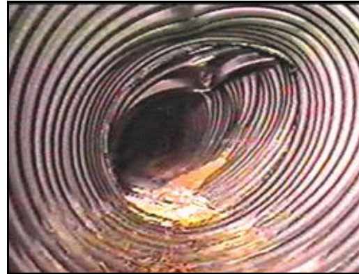
Figure 99. — HDPE pipe experiencing extensive shape deformation.
