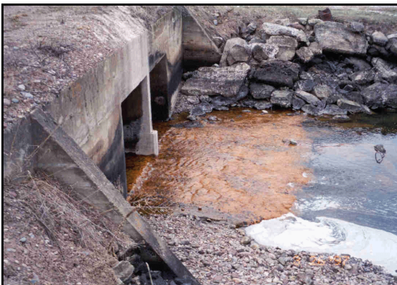
Figure 44. —The outlet shows an example of biofouling.
