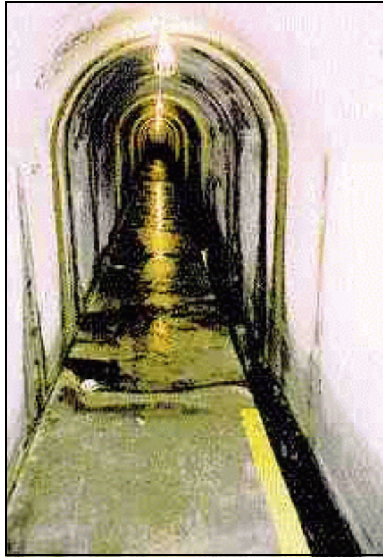
Figure 112. —Iron sulphide deposits in foundation gallery.
