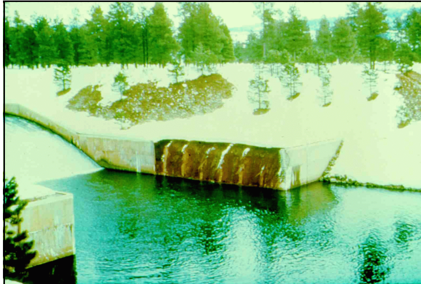
a. Vallecito Dam spillway stilling basin, Colorado.—Failure of the left retaining wall was the result of inadequate drainage provisions, which led to accumulation of water behind the wall, and subsequent large lateral loads, due to ice formation.
