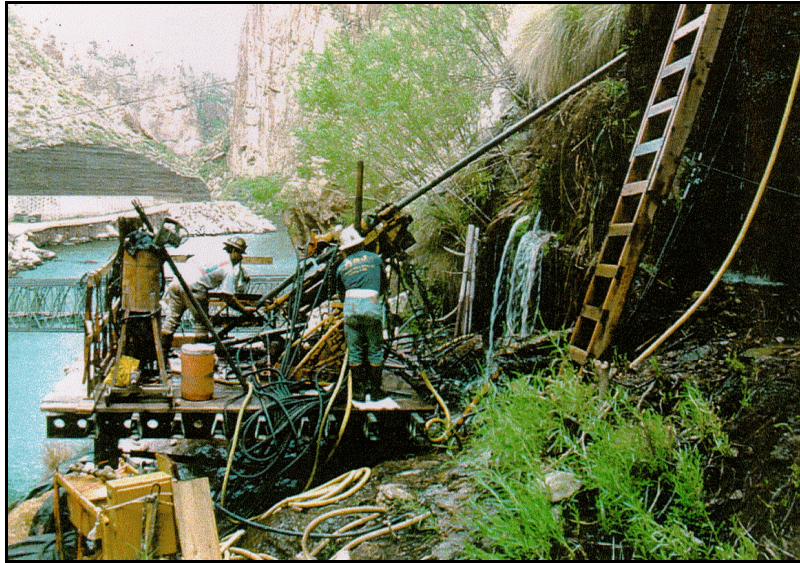
Figure 44. —View of rotary drilling operations to install high-angle drain holes in bedrock from a platform on the downstream right abutment of Horse Mesa Dam, Arizona. The drill rig is a Craelius Diamec 260.
