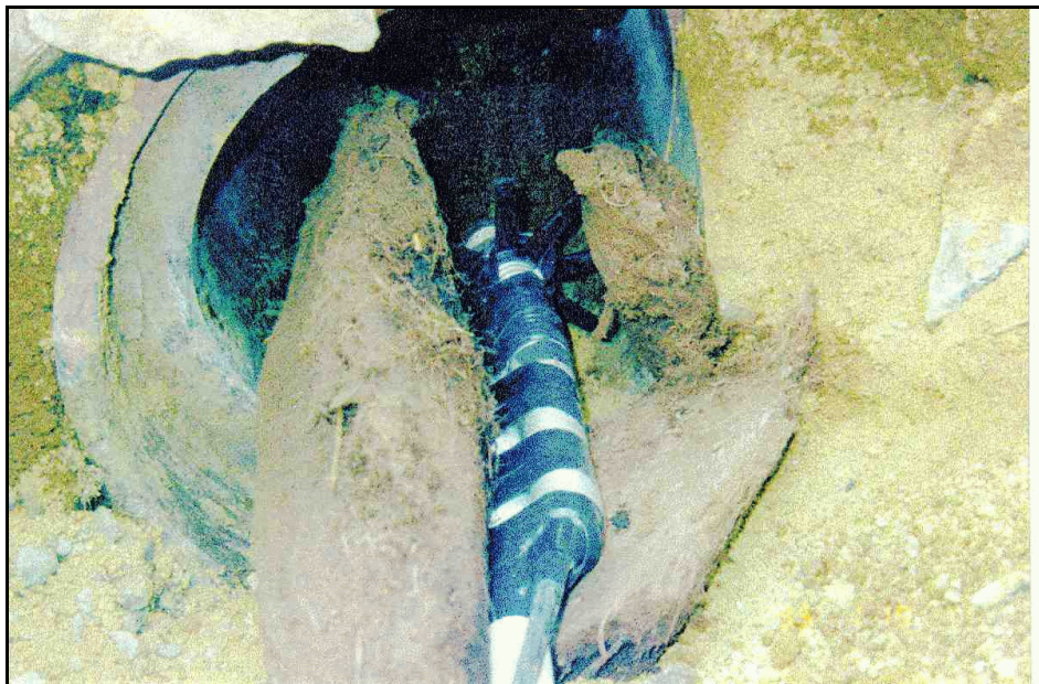
Figure 113. —Plug of organic material in toe drain (also shown is camera used to inspect drain).
