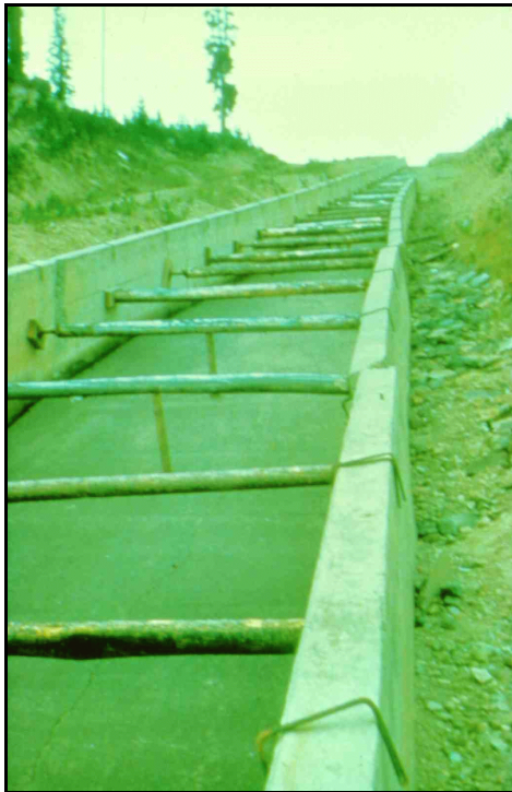
d. Grassy Lake Dam spillway, Wyoming.—Due to excessive frost heave, walls have failed.
