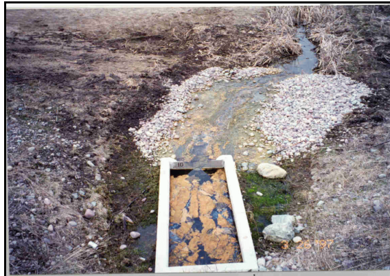
Figure 46. —The weir shows an example of biofouling.
