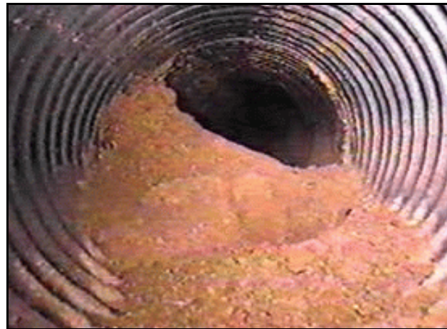
Figure 101. —An HDPE pipe joint has experienced extensive separation. Materials surrounding the pipe have entered through the separated joint.
