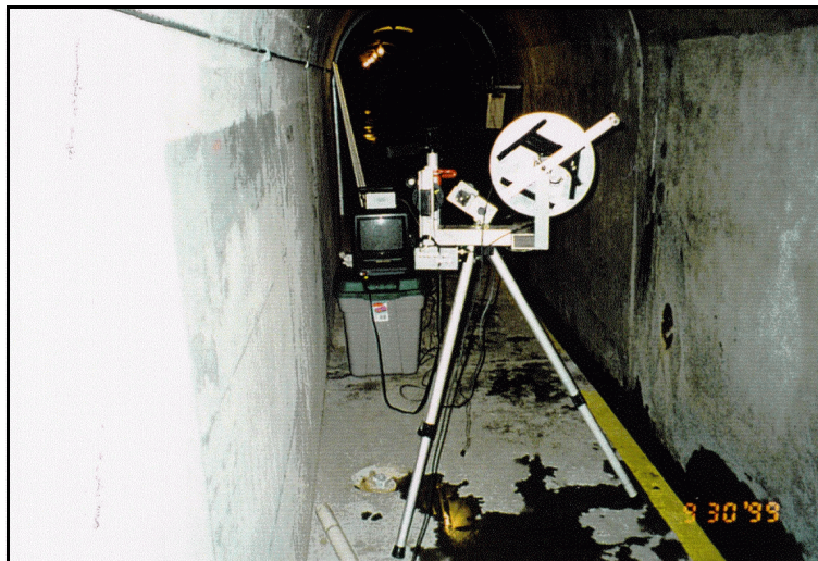
Figure 41.—Down-hole video equipment used to determine the condition of the drains before and after cleaning.
