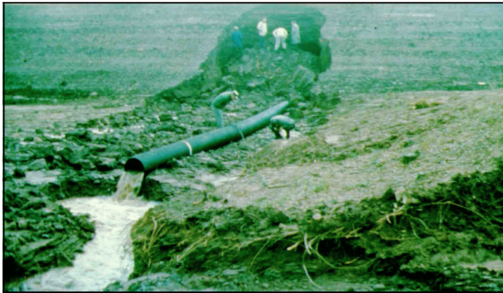
f. Unknown dam.—The worst-case scenario for piping of adjacent embankment material can lead to failure of not only the outlet works, but also the embankment.
