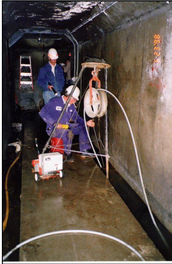
Figure 114.—High pressure water jet nozzle and hose being lowered into foundation drain.
