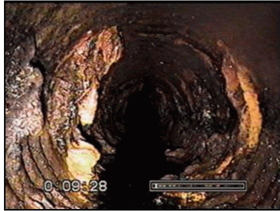
Figure 51. —Calcium carbonate precipitate was observed covering the 18-inch pipe interior about 60 ft upstream of the outfall exit portal of a toe drain.
