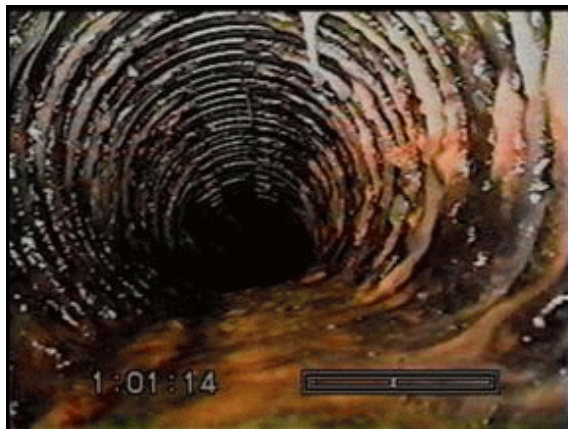
Figure 47. —The bacterial growth is partially covering the inside of 8-inch diameter HDPE pipe.
