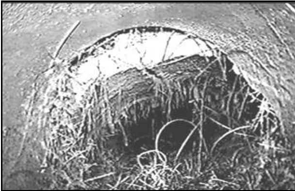
Figure 98. — Clay tile pipe experiencing inward collapse of the crown.
