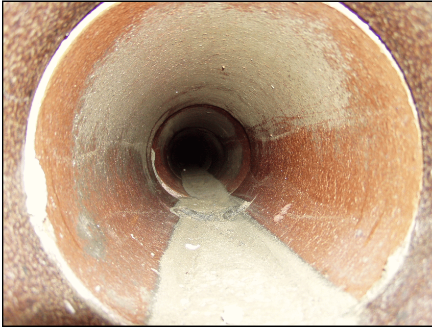
Figure 92.—Clay tile outfall pipe with fines in the invert.
