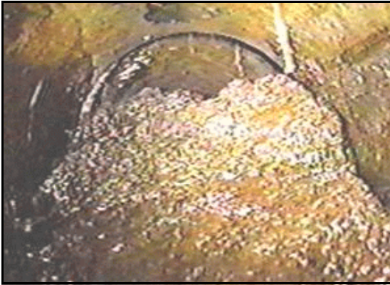
Figure 107. —Accumulation of sediments has resulted in plugging of the pipe.
