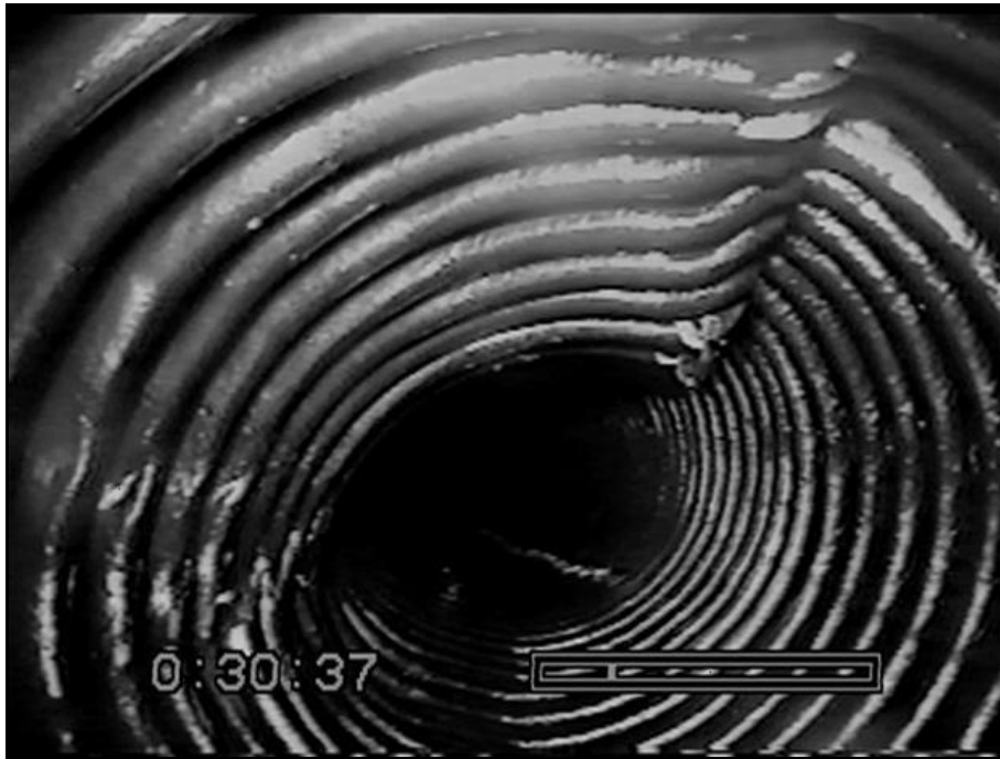
Figure 90. —A damaged left toe drain pipe at approximately sta. 23+25 stopped the camera-crawler. A cleaning removed fine materials from the pipe invert.
