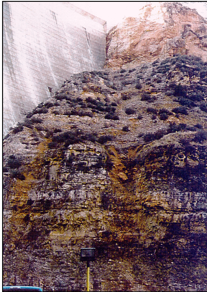
Figure 2. —Madison Limestone outcrop in the left abutment downstream from the dam. Note the weathering in fractured zones. The rock in this abutment is not as sound as in the other abutment.
