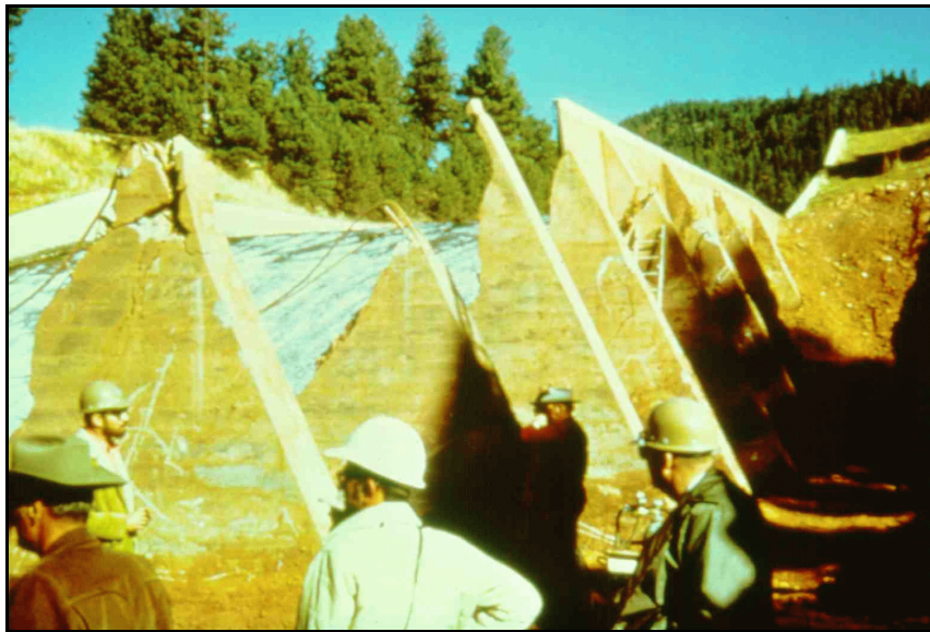
b. Vallecito Dam spillway stilling basin, Colorado.—After backfill was excavated, only portions of the counterforts remained.
