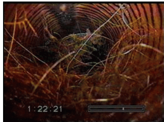
Figure 53. —Vegetative growth shown fouling 8-inch-diameter HDPE pipe.
