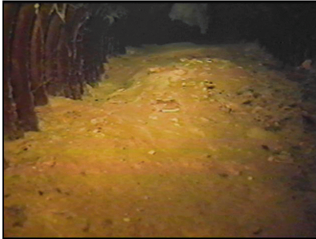
Figure 21. —Example of sediment deposition encountered during a video inspection of a toe drain.
