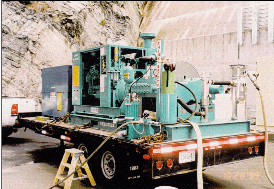
Figure 27. —High pressure water jetting unit used to clean drains. Pump powered by a 215-hp diesel engine.
