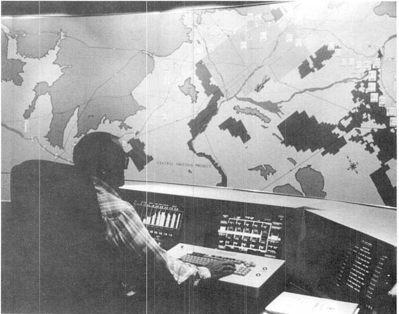
Figure 3-18. — Typical master station control console.
