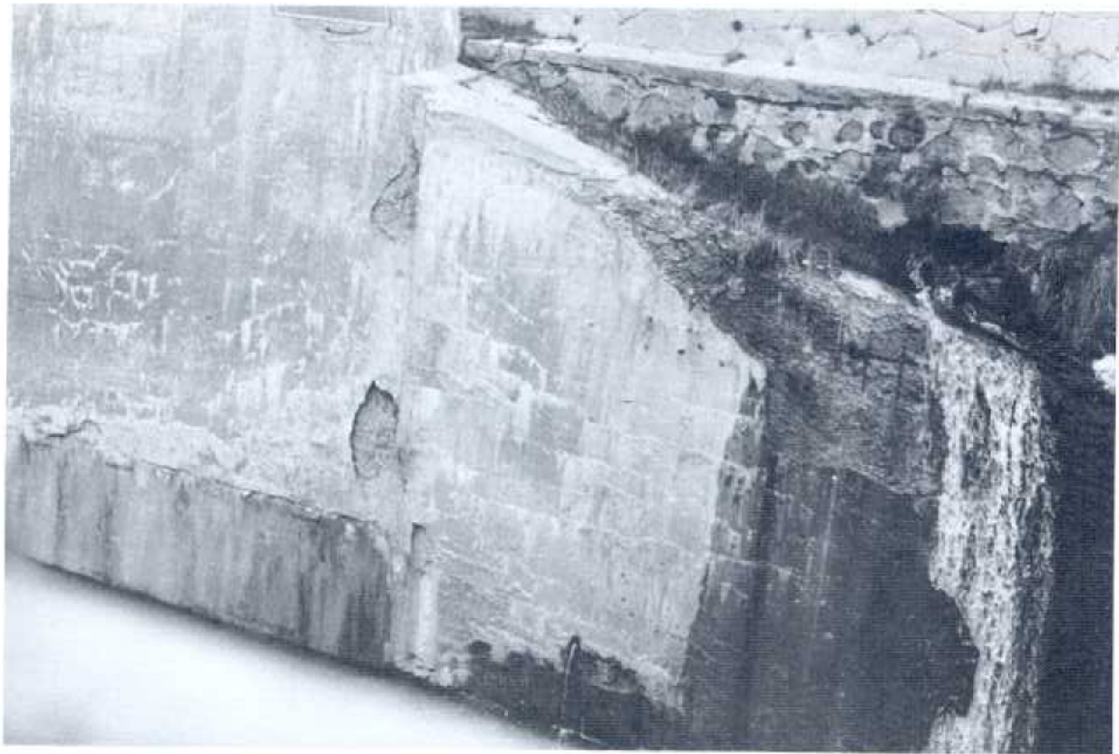
Figure 5-7.—Island Park Dam, closeup of spillway damage. P-801-D-79388.
