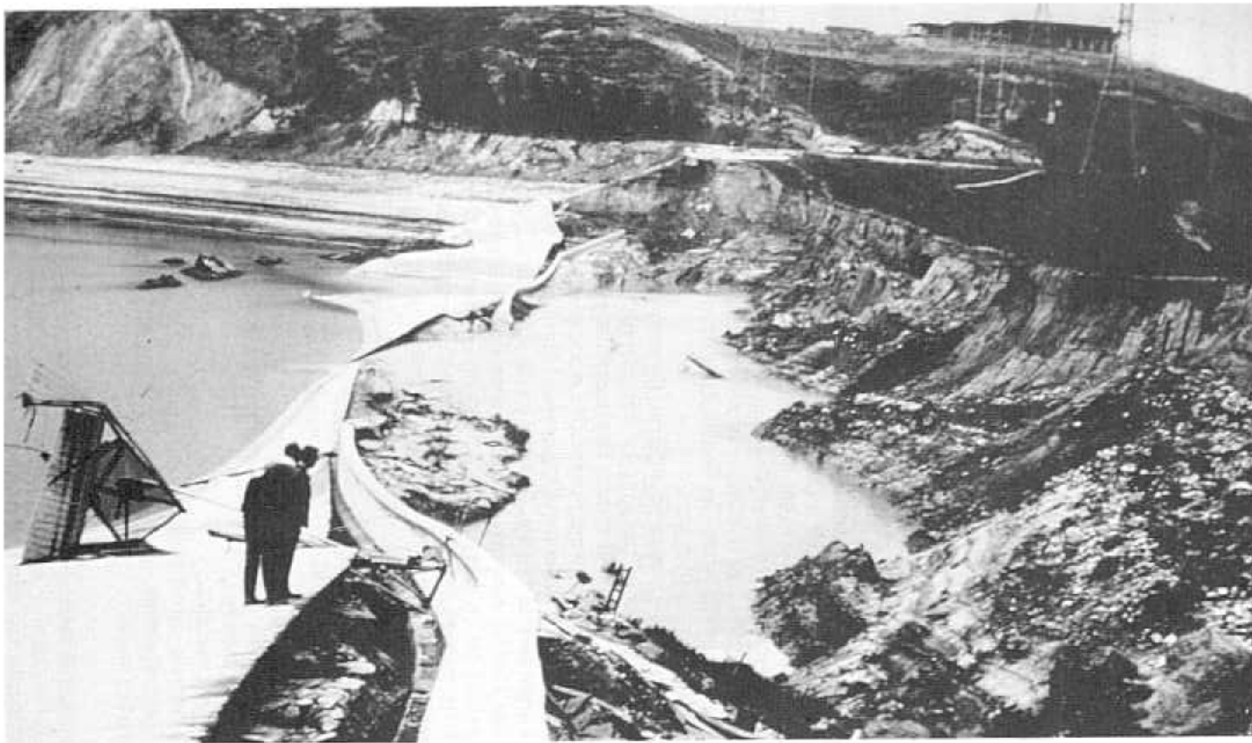
Figure 5-2. Upstream face of Lower Van Norman (San Fernando) Dam after failure (Courtesy, Calif. Dept. of Water Resources). P-801-D-79383.
