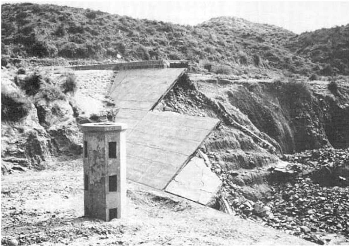
Figure 4-6.—Frías Dam after failure, upstream view (Courtesy of C. J. Cortright). P-801-D-79351.
