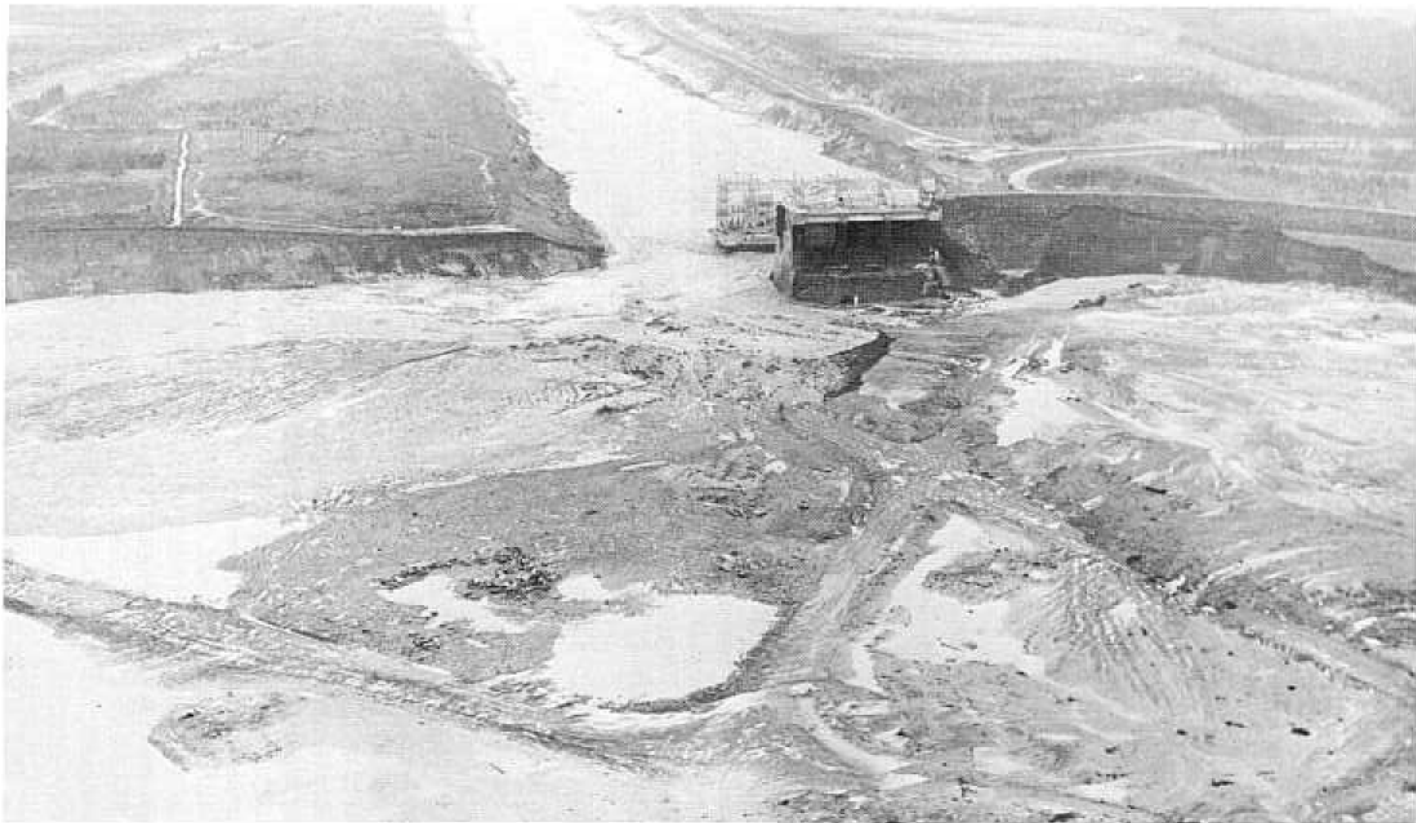
Figure 4-29.—Walter Bouldin Dam after failure (Courtesy, The Alabama Power Company). P-801-D-79381.
