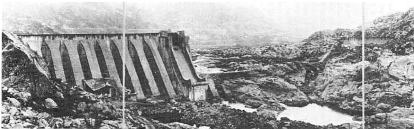
Figure 4-28.—Vega de Tera Dam after failure (Courtesy, Comité Nacional Español, ICOLD). P-801-D-79380.
