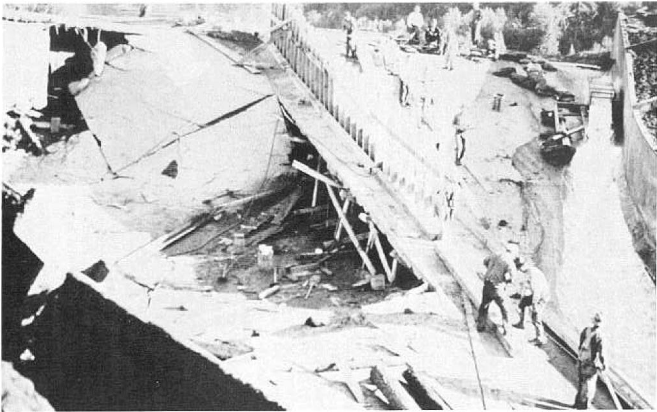
Figure 5-8.—Damaged spillway on embankment—Middle Fork Dam (Courtesy, Calif. Dept. of Water Resources). P-801-D-79389.
