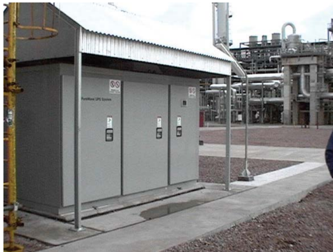
Figure 32. PureWave UPS system installed at a continuous process manufacturing plant
