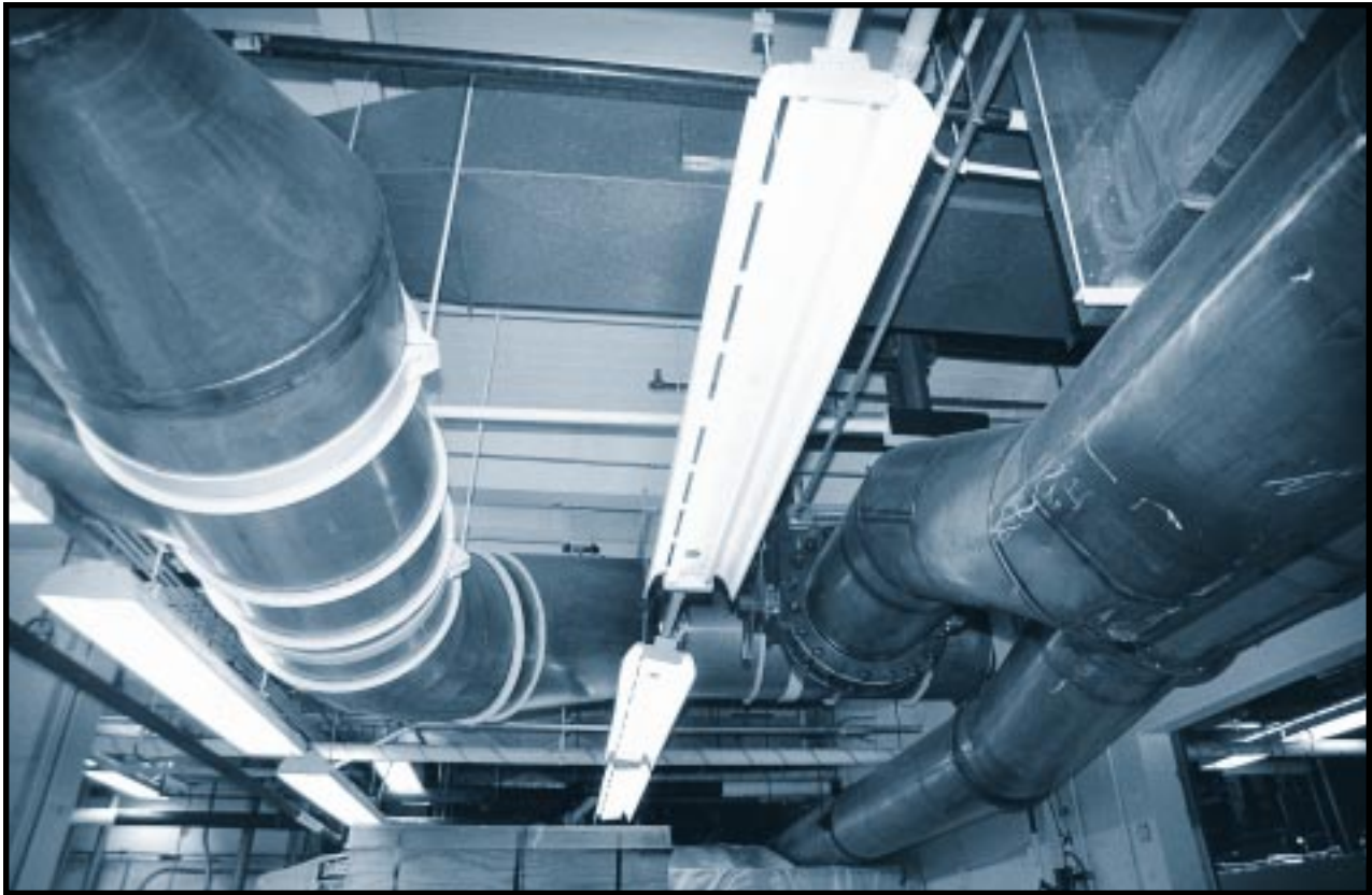
Ventilation ducts contaminated with plutonium in dust, oxides, and smoke exhausted from gloveboxes in the pyrochemistry area of Rocky Flats. When a buildup of plutonium becomes too great, it can pose a criticality threat. The buildup in these ducts was close to the limit for such a threat. Building 776, Rocky Flats Plant, Colorado. December 20, 1993.
