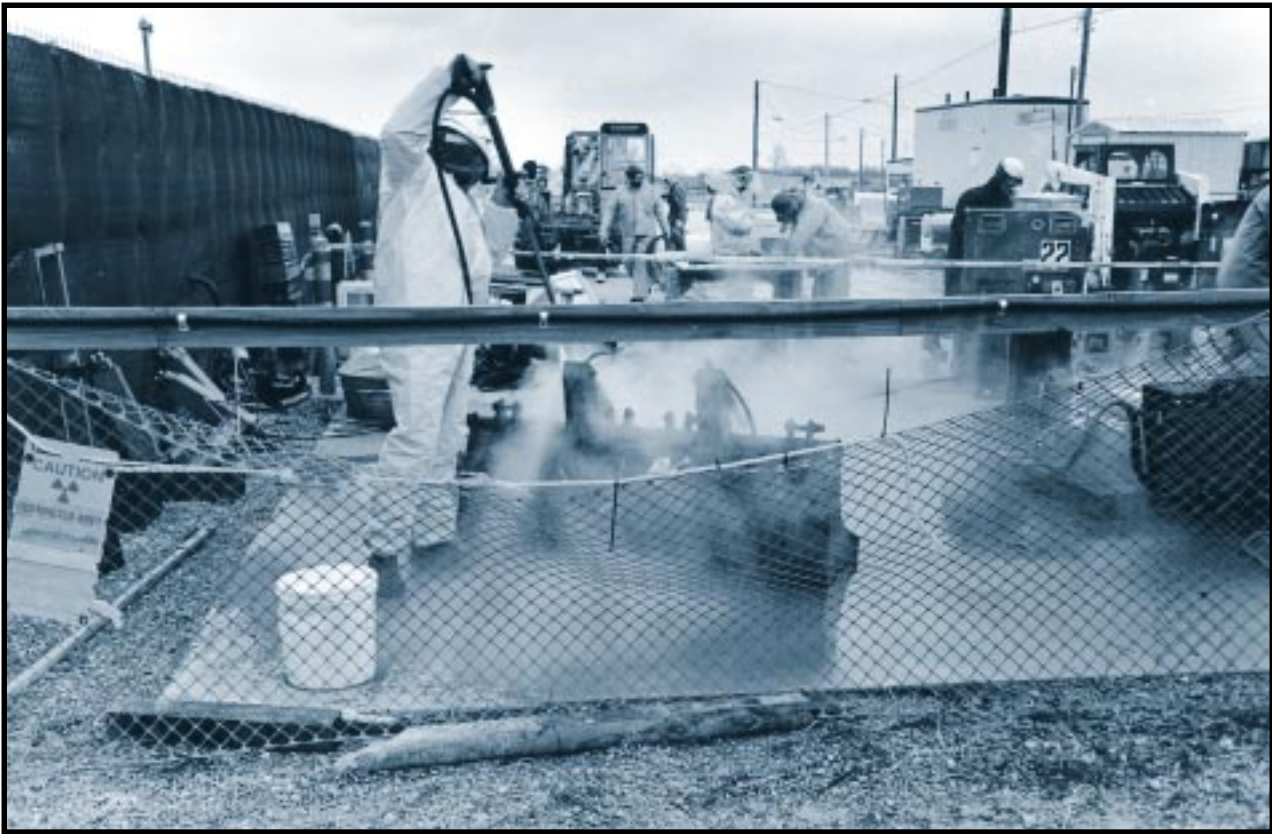
Workers are decontaminating equipment used to move contaminated soil at the Weldon Spring site. Facilities at this site once performed many of the same functions as the Fernald Plant. Weldon Spring site, Missouri. January 29, 1994.
