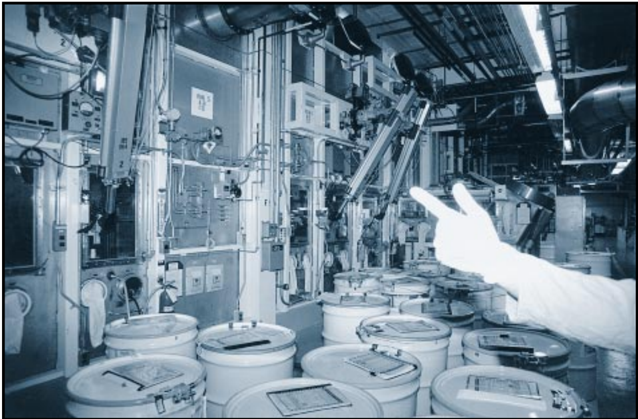
Some barrels of residues from plutonium operations are stored in drums in the building in which they were processed. Building 776/777, Rocky Flats Plant, Colorado. December 20, 1993.
