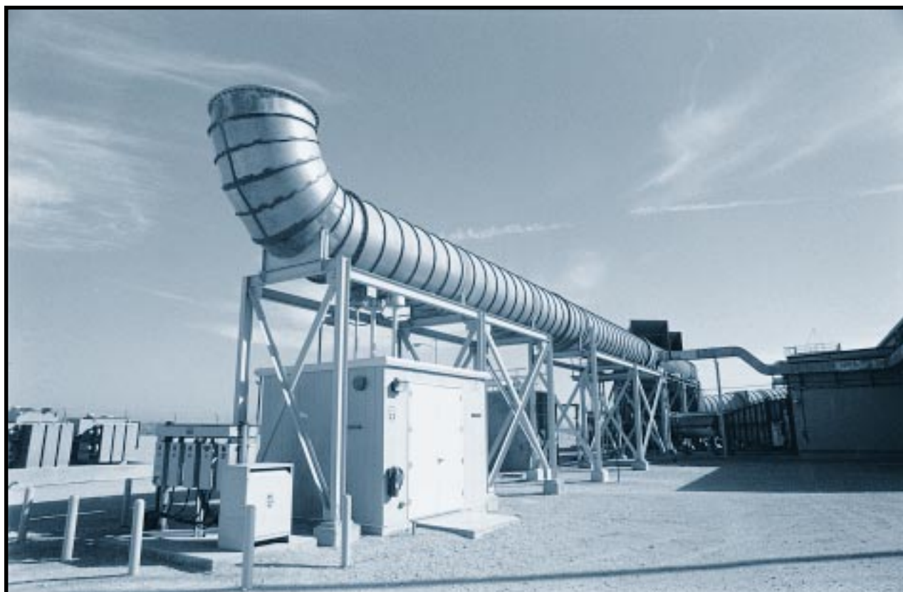
Emergency exhaust airway at the WIPP. Should an accidental release of radiation occur within the WIPP's system of underground chambers, exhaust ventilation air would be diverted through a bank of filters to clean the air before it is released through this duct. Waste Isolation Pilot Plant, Carlsbad, New Mexico. February 25, 1994.
