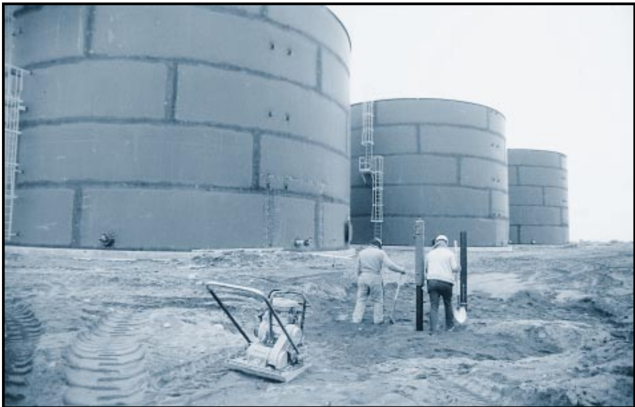
A wastewater-treatment facility under construction at Hanford to treat low-level condensate from an evaporation process that reduces the volumes of high-level waste. Each of these three tanks has a capacity of 670,000 gallons. Because of the use of this facility, the Department has ceased discharges of contaminated waste water to the soil for the first time in more than 40 years. Hanford Site, Washington. December 19, 1993.
