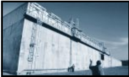
12. To store the waste from the Saltstone Facility, we built the grout vaults.
