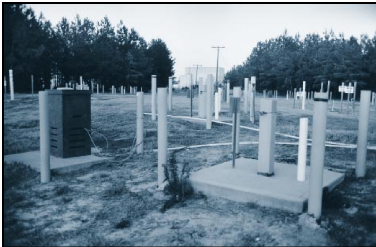
The Integrated Demonstration Site at the Savannah River Site contains 150 monitoring wells, some quite shallow, some as deep as 200 feet. These wells are used to chart the migration of contaminants through the water table and through different levels of soil and rock. Included within this site is the world's first horizontal injection well used for environmental remediation. A-M Area, Savannah River Site, South Carolina. January 6, 1994.
