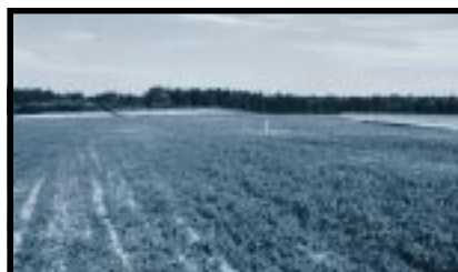
7. To arrest spreading ground-water contamination from waste poured into the seepage basins, we built clay caps over them and installed pumping wells.
