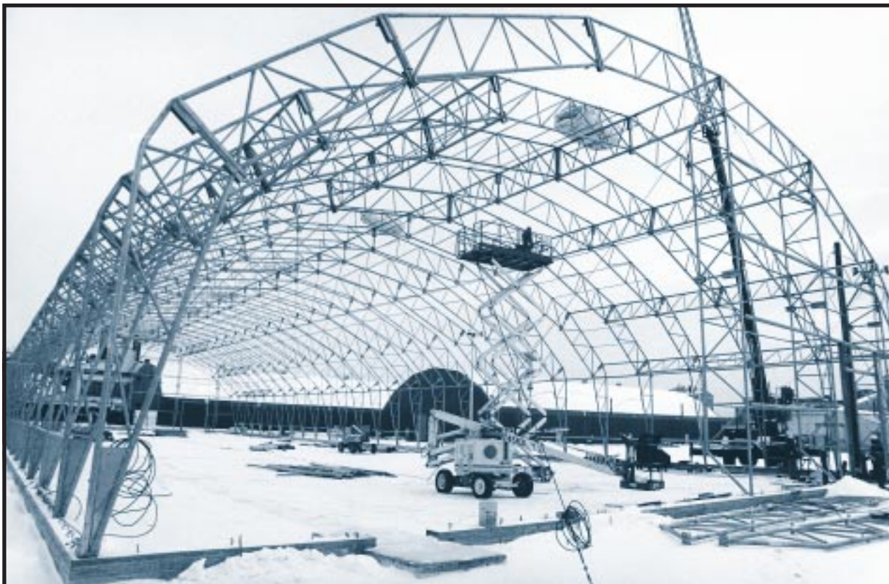
A temporary tension-support structure is being constructed at Fernald. These lightweight structures are increasingly used throughout the former nuclear weapons complex. They keep drums of various types of waste out of the elements, extending their storage life at relatively low cost. Plant 1 pad, Fernald Environmental Management Project, Fernald, Ohio. December 28, 1993.
