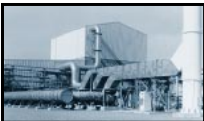
8. To provide an alternative for discharging effluent from the evaporators, we built the Effluent Treatment Facility.
