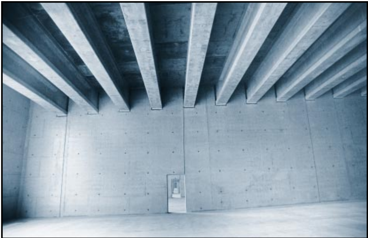
This new vault for storing low-level waste contains 12 large cells, each of them 55 feet long, 150 feet wide, and 30 feet high. The first facility of its kind in the country, this vault system will replace shallow burial in engineered trenches at the Savannah River Site. This vault began storing waste in September 1994. Once full, it will be covered with clay to form a mound with a plant cover. E Area Vault, Solid Waste Management Division, Savannah River Site, South Carolina. January 7, 1994.
