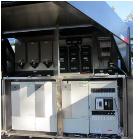
Figure 4. Components mounted in a NEMA 4X enclosure in the front of the trailer include (clockwise from top left) combiner boxes and charge controllers, breakers to loads, and inverters. Photo: Alicen Kandt
