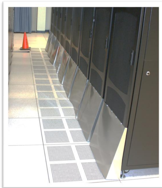
Figure 3. Hoods for Power Supply Unit Air Intake
