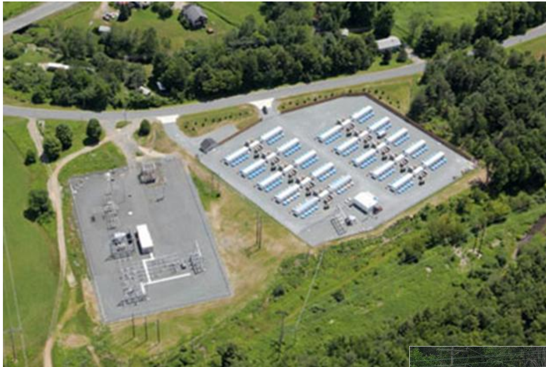
20 MW flywheel system operating in NYISO
