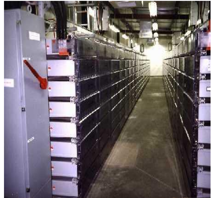
Critical Load Backup/ Energy Management Lead Smelter: Battery Recycling 5 MW, 3.5 MWH VRLA Battery
