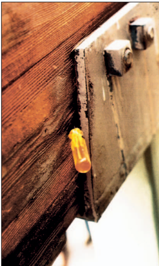
Figure 14-2. Wood decay behind a metal beam connector
