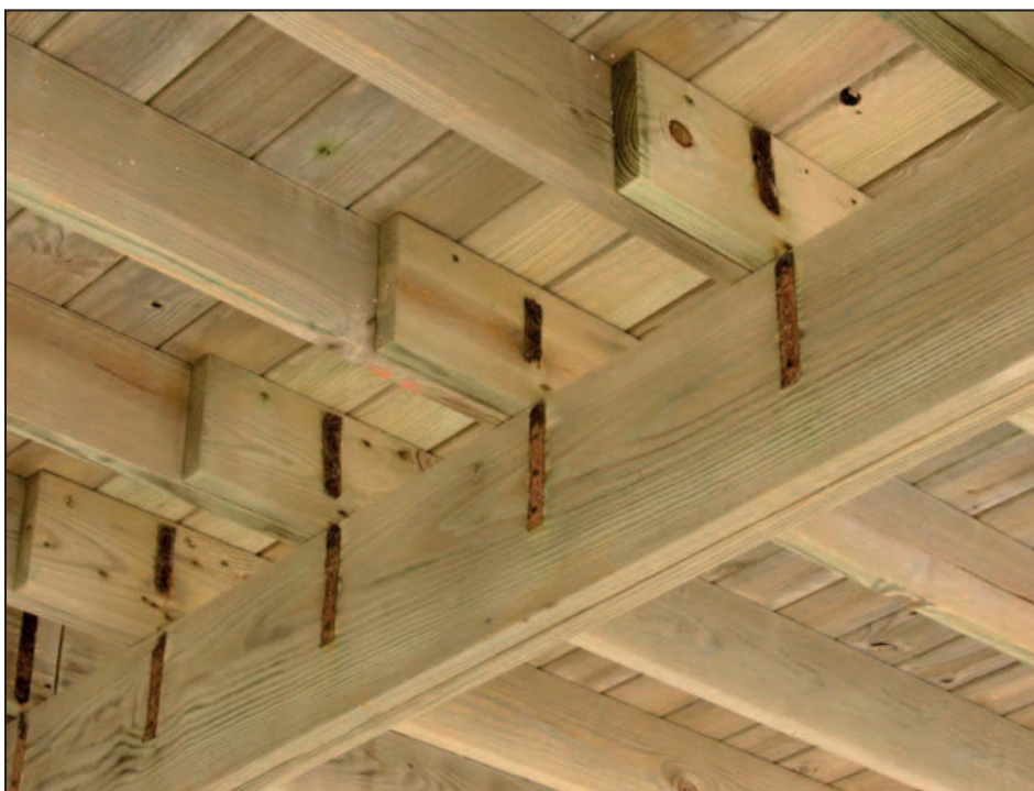
Figure 14-3. Severely corroded deck connectors
