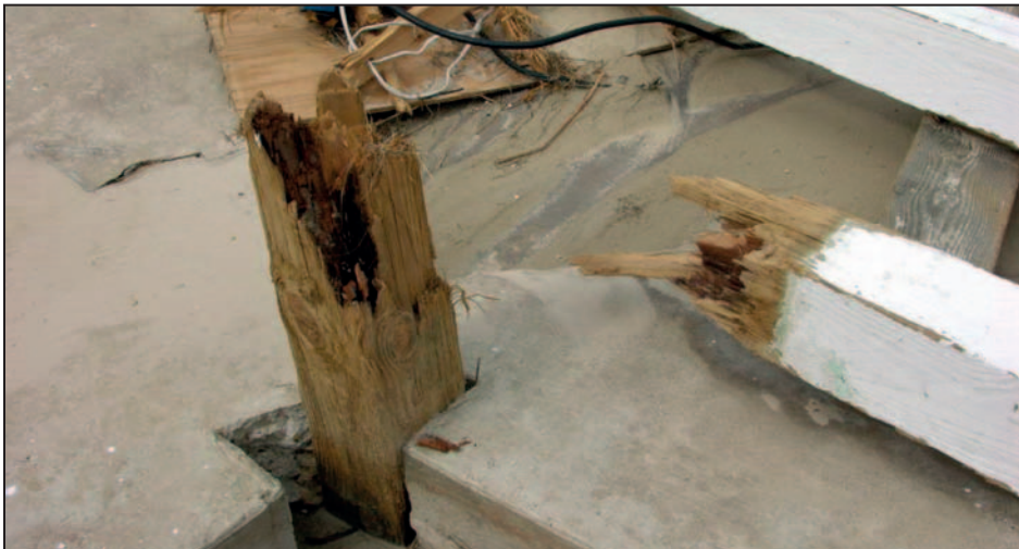
Figure 14-1. Pile that appears acceptable from the exterior but has interior decay
