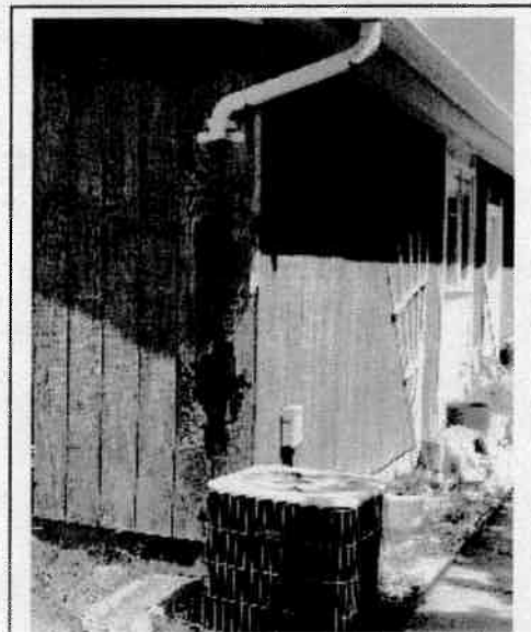
Figure 5. Gutter System - The missing downspout has led to severe rotting of the siding materials.
