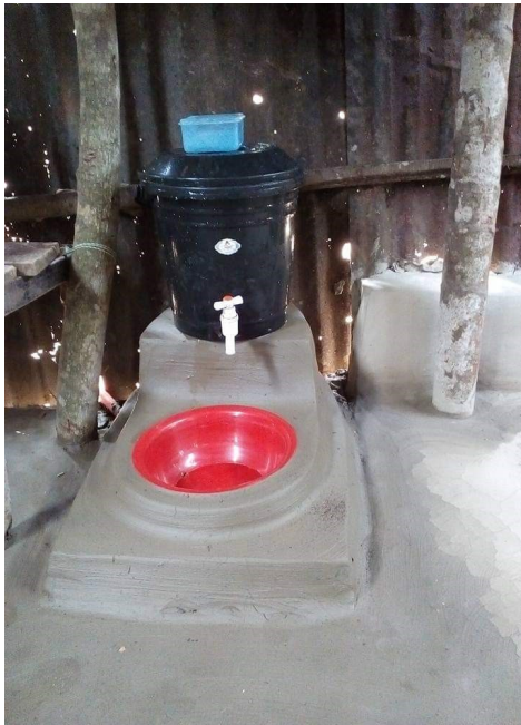
Bucket with tap, installed inside the kitchen along with plastic bowl for basin
