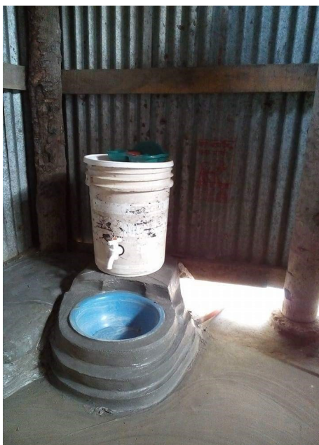
Used paint container with tap and installed inside the kitchen along with plastic bowl for basin
