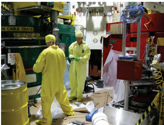
Paul Liposky and Jim Moody work on the RT-4 pneumatic transfer system.
