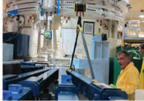
▲ Mike Rinehart and Doug Ogg (l-r) re-install the NG-1 vacuum jacket in C-100. The first guide elements of existing guides NG-1 thru 7 were replaced as part of the refurbishment program.
