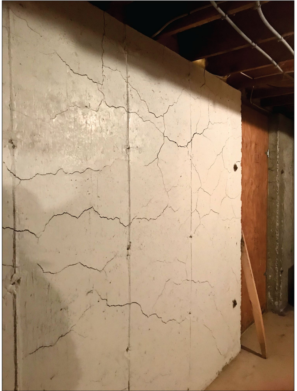
Figure 2: Basement with Severe Pyrrhotite Damage
