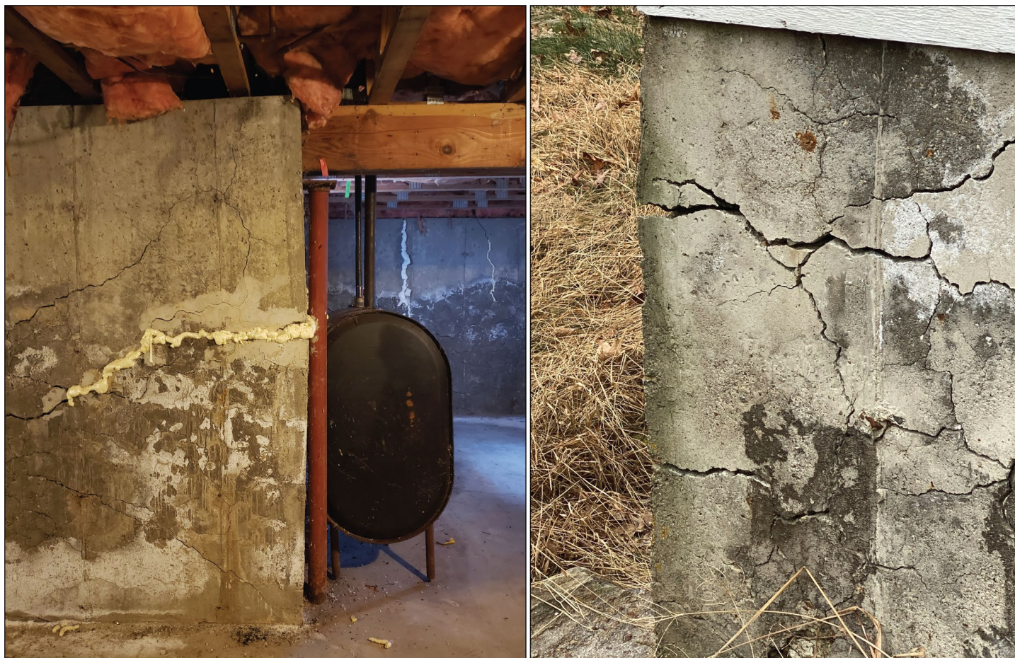
Figure 3: Basement and Exterior of a Home Condemned Due to Pyrrhotite Damage
