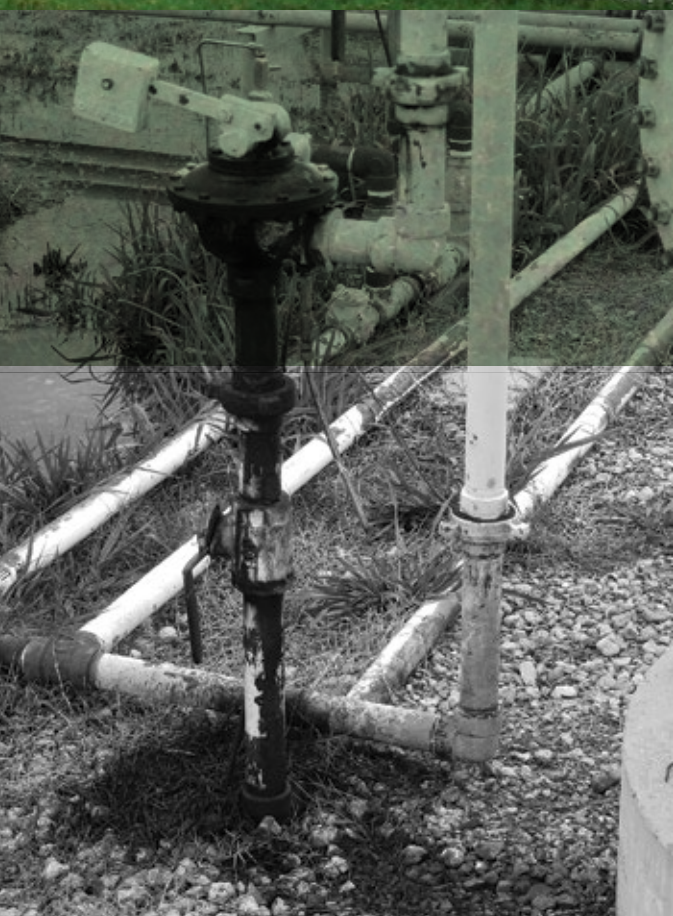
Flowlines cross a mudflat at San Bernard National Wildlife Refuge in Texas. Some flowlines are abandoned and corroded.
