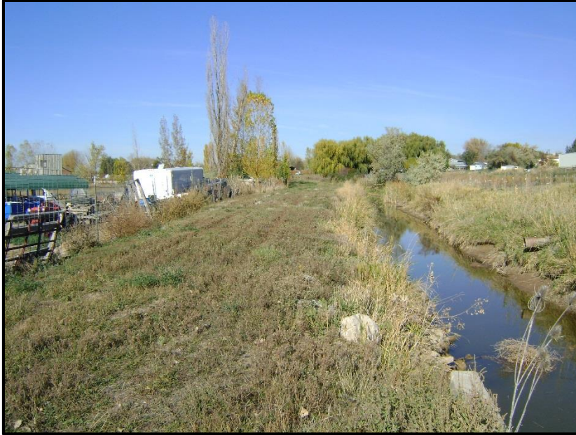
Photo 1: Looking easterly at the southernmost section of the Davis and Weber Canal that is contained within the project action area. This section of the canal is currently unlined.
