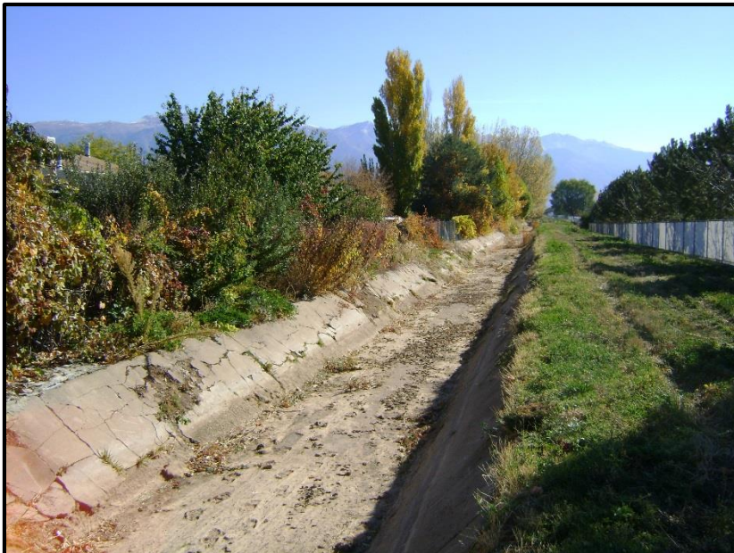
Photo 2: Looking easterly at a portion of the canal that is lined, but has deteriorated significantly. This photo was taken near the intersection of 2450 North and 1100 West.
