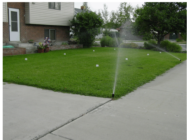
Figure 6 Sprinkler system performance test in progress
