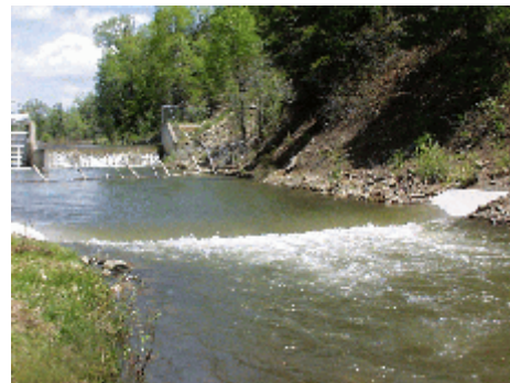
Ramp flume constructed in the Florida River below Florida Farmers Diversion Dam.
