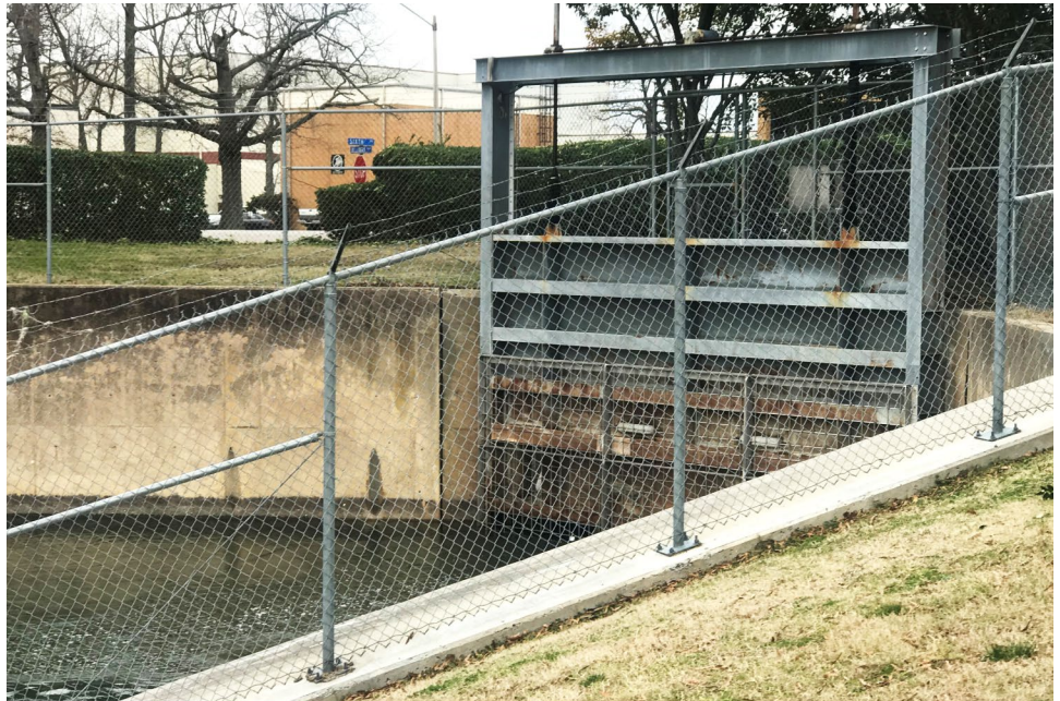
Figure 4: Flood Control Gate, Naval Station Norfolk, Virginia
