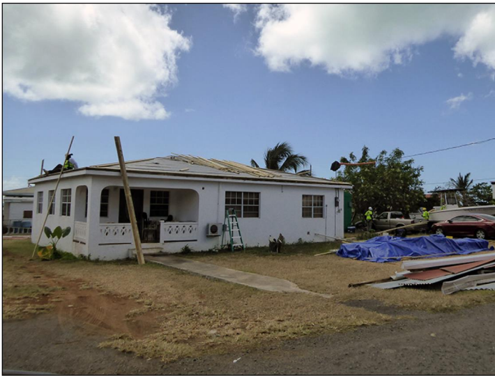
Home undergoing permanent roof replacement through Phase II of the STEP pilot program.
