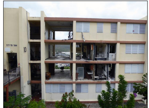
Hurricane force winds completely destroyed apartments in a public housing facility in St. Thomas.
