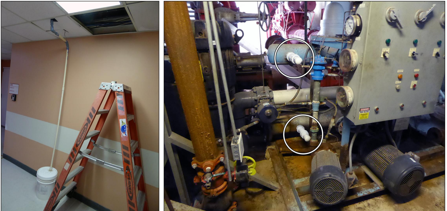
Figure 18: Examples of Temporary Fixes to the Governor Juan F. Luis Hospital and Medical Center as of March 2019, St. Croix, U.S. Virgin Islands
