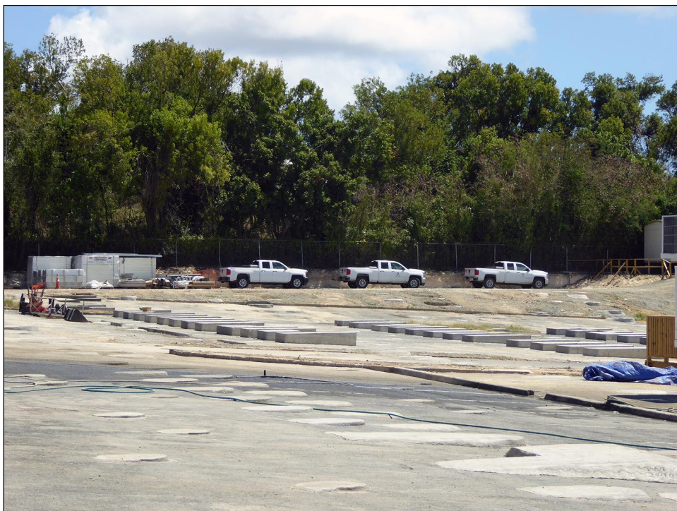
Figure 17: Future Location of the Governor Juan F. Luis Hospital and Medical Center Temporary Facility as of March 2019, St. Croix, U.S. Virgin Islands
