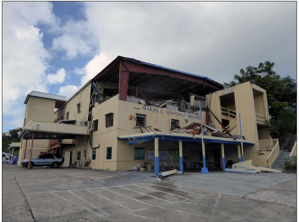
Figure 4: Hurricane Damage to the Virgin Islands Housing Authority’s Central Office as of October 2018, St. Thomas, U.S. Virgin Islands
