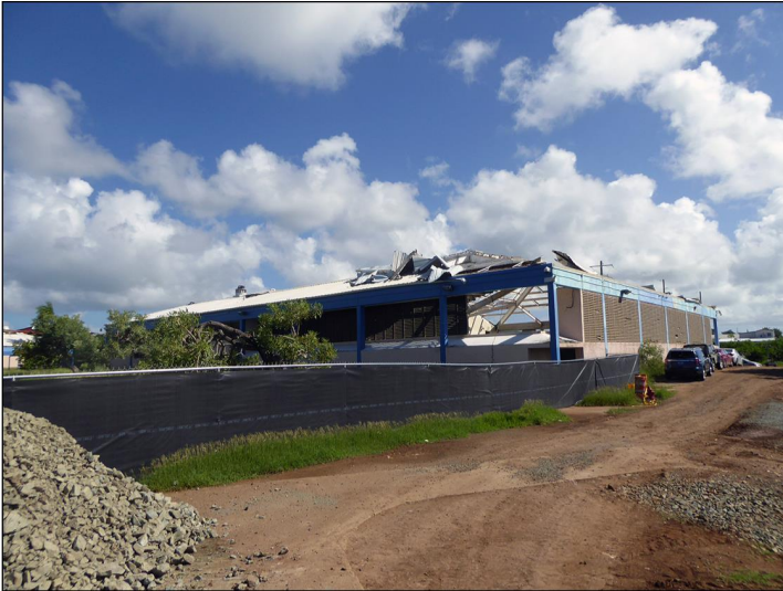
This school building in St. Croix sustained severe hurricane damage, including a collapsed roof.
