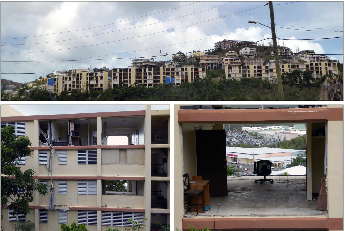
Figure 11: Examples of Hurricane Damage to a Public Housing Facility in St. Thomas, U.S. Virgin Islands
