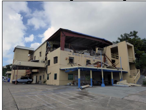
The Virgin Islands Housing Authority office in St. Thomas sustained significant damage during the storms.
