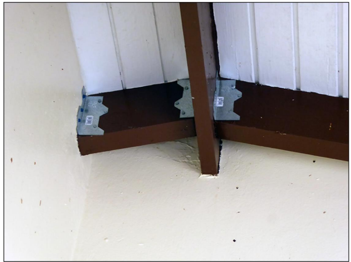
Home with completed permanent roof replacement through Phase II of the STEP pilot program, which included the installation of hurricane clips to increase the roof’s resiliency during hurricane-strength winds.
