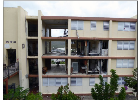
Hurricane force winds completely destroyed apartments in a public housing facility in St. Thomas.
