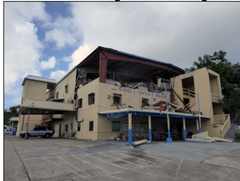
The Virgin Islands Housing Authority office in St. Thomas sustained significant damage during the storms.
