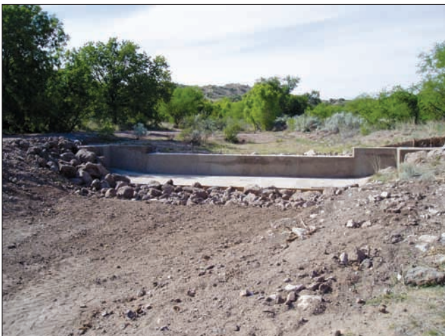
Figure 8. The fish barrier on Sonoita Creek, Santa Cruz County, Arizona, downstream from Cottonwood Spring.
