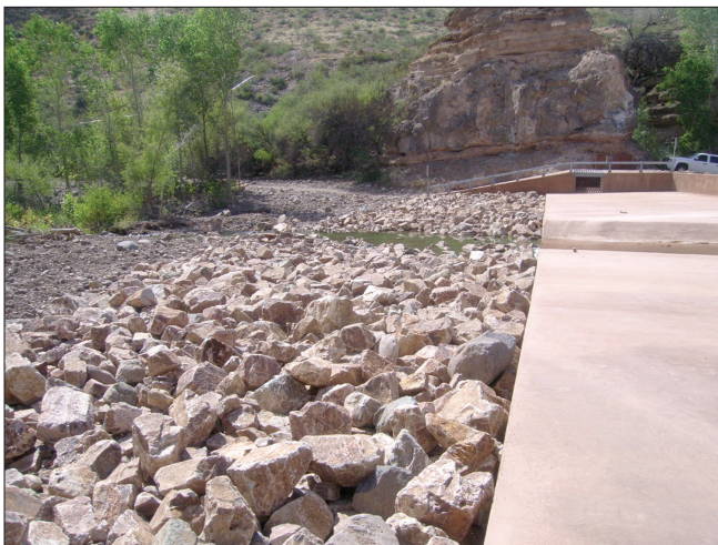
Figure 3. Riprap placement downstream from the apron of the Bonita Creek fish barrier, Graham County, Arizona.
