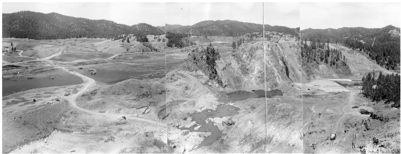
Early construction of Pactola Dam in 1954 as seen from the location of the present day Visitors Center. The name Pactola comes from the Greek word Pactolus meaning “gold-bearing sands”.
