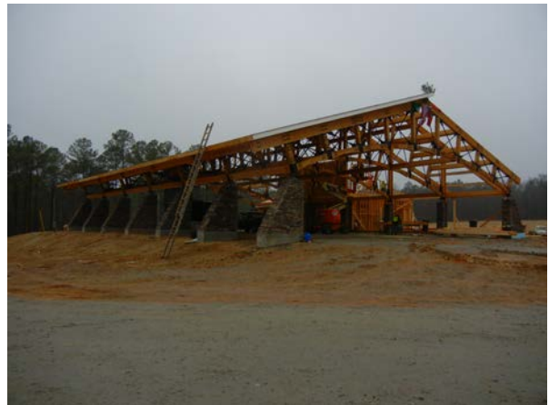
Construction of Palmetto Shooting Complex – SC Credit: SC Department of Natural Resources
