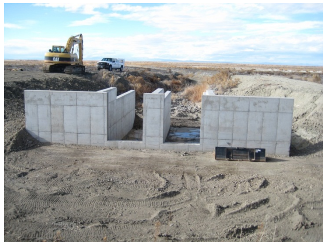
Deferred maintenance project at Stillwater NWR, NV: Above picture shows project to replace water control structure in progress.
