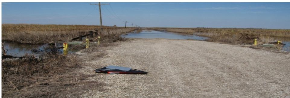
Washed out road at Anahuac NWR, TX. The Fish and Wildlife Service Transportation Program provides funding to maintain public use roads, bridges, and parking areas.
