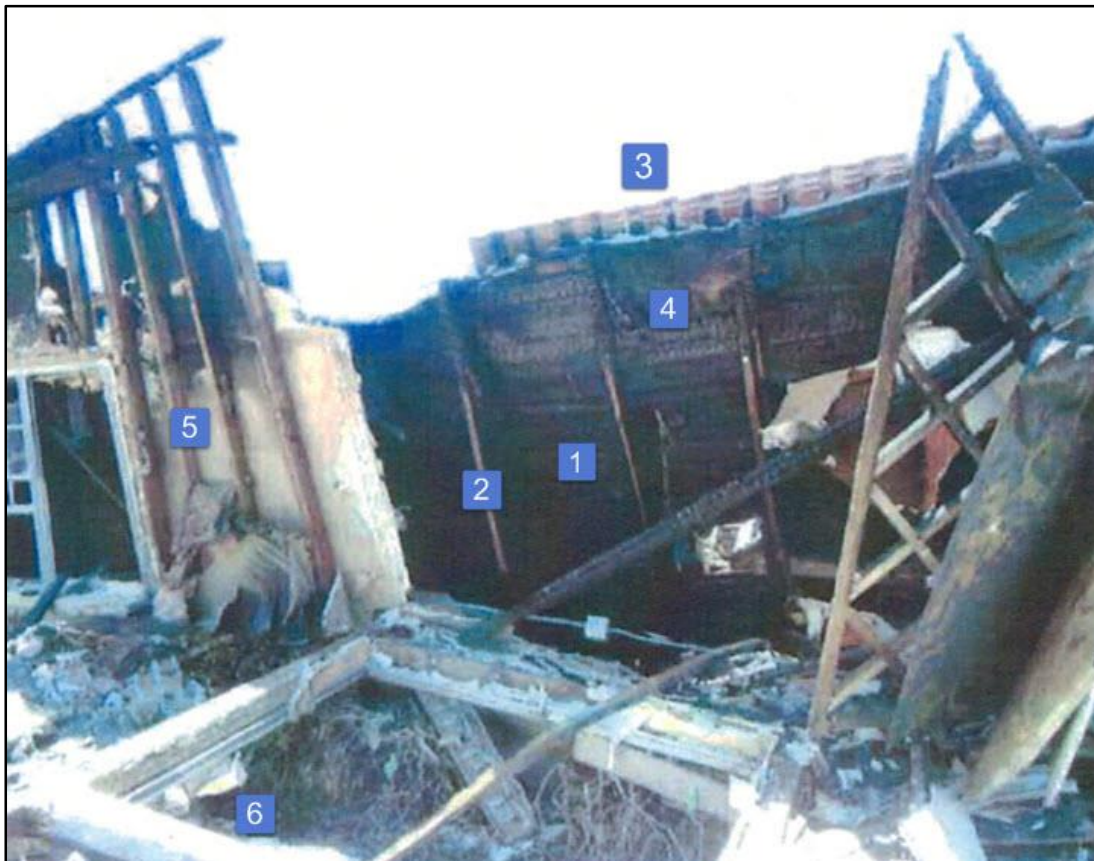
Photo 1. View of Division Alpha Perimeter Wall & Lean-To Roof Collapse (Fire Department Photo/ Diagram Courtesy of Buildingsonfire.com)
