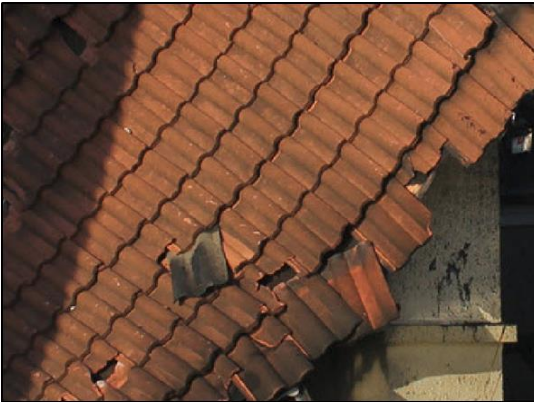
Photo 2. Concrete Roofing Tiles - Post Fire (NIOSH Photograph)
