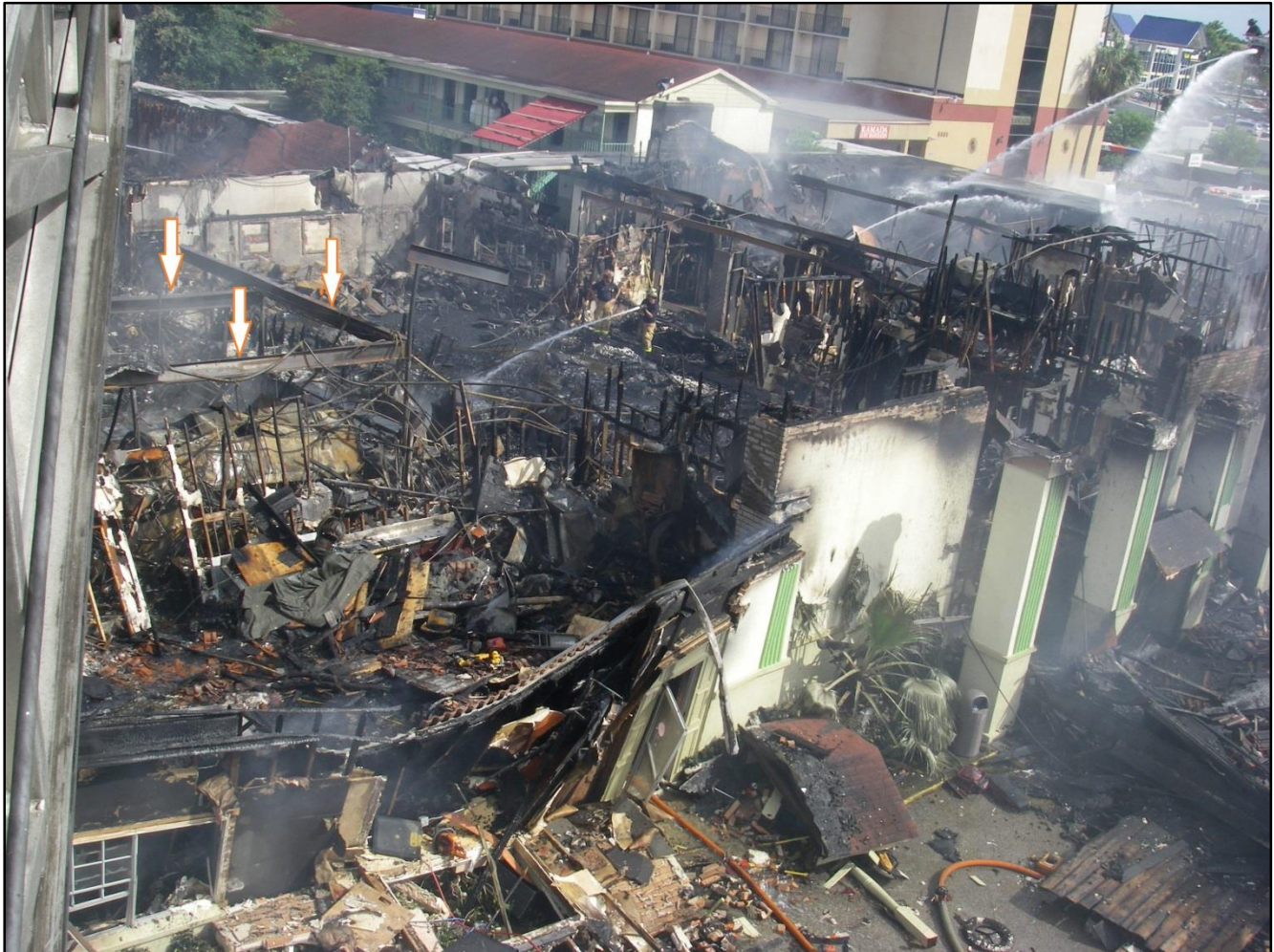
Photo 4. The arrows indicate the support system for the 2 nd floor and void space above the restaurant and lobby area of the motel.
