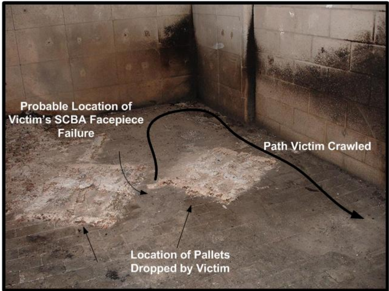
Photo 3. Basement Burn Room after Incident.
