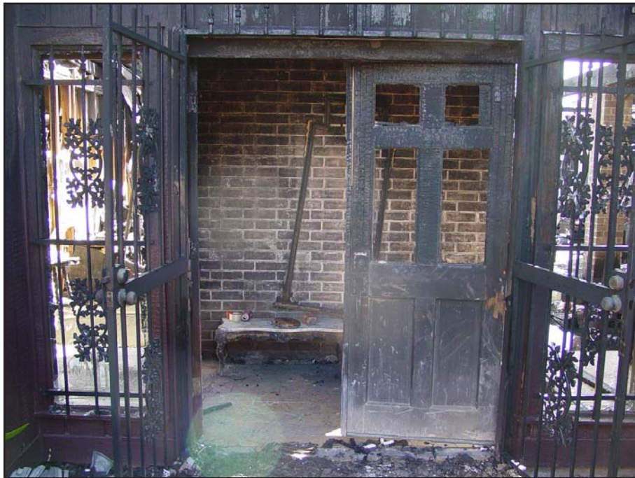
Photo 1. Illustrates the front door (side-A) and the burglar bars restricting entry. Note that this security measure was on every access door and window of the structure
