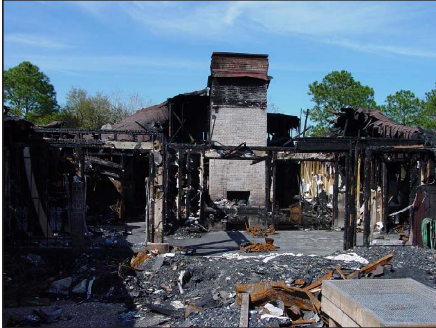
Photo 2. Depicts the rear (side-C) of the structure. Note the collapse area included the majority of the structure, including around the chimney near where the victim was found.
