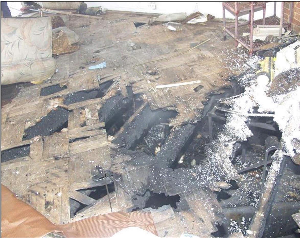
Photo 2. Floor area consumed by fire
