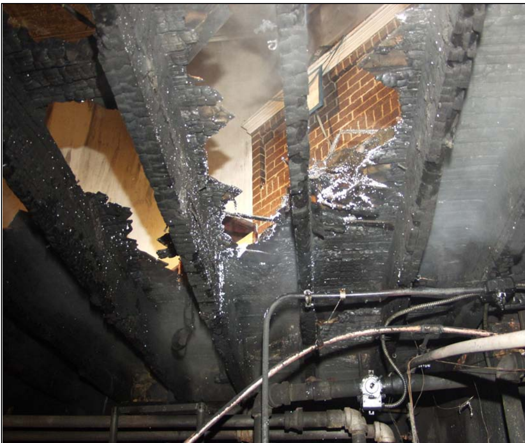
Photo 3. View from basement of floor area consumed by fire
