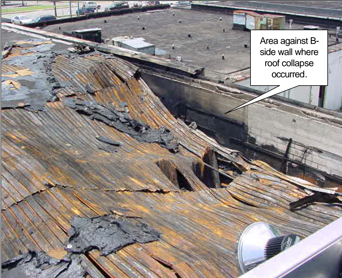
Photo 2. Roof collapse B-Side
