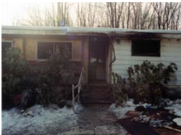
Mobile Home Involved in Fire
