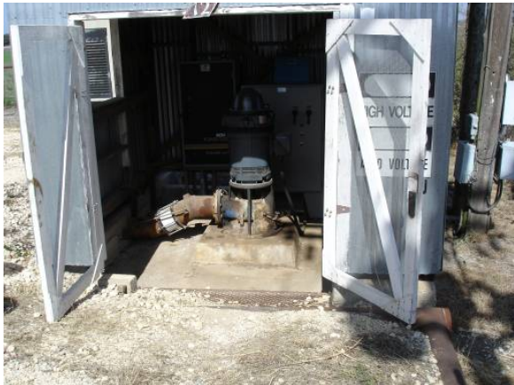
Figure B10c: Well house and power head for Burkett Well (to be refurbished).
