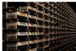
HPSS Back-up Storage
