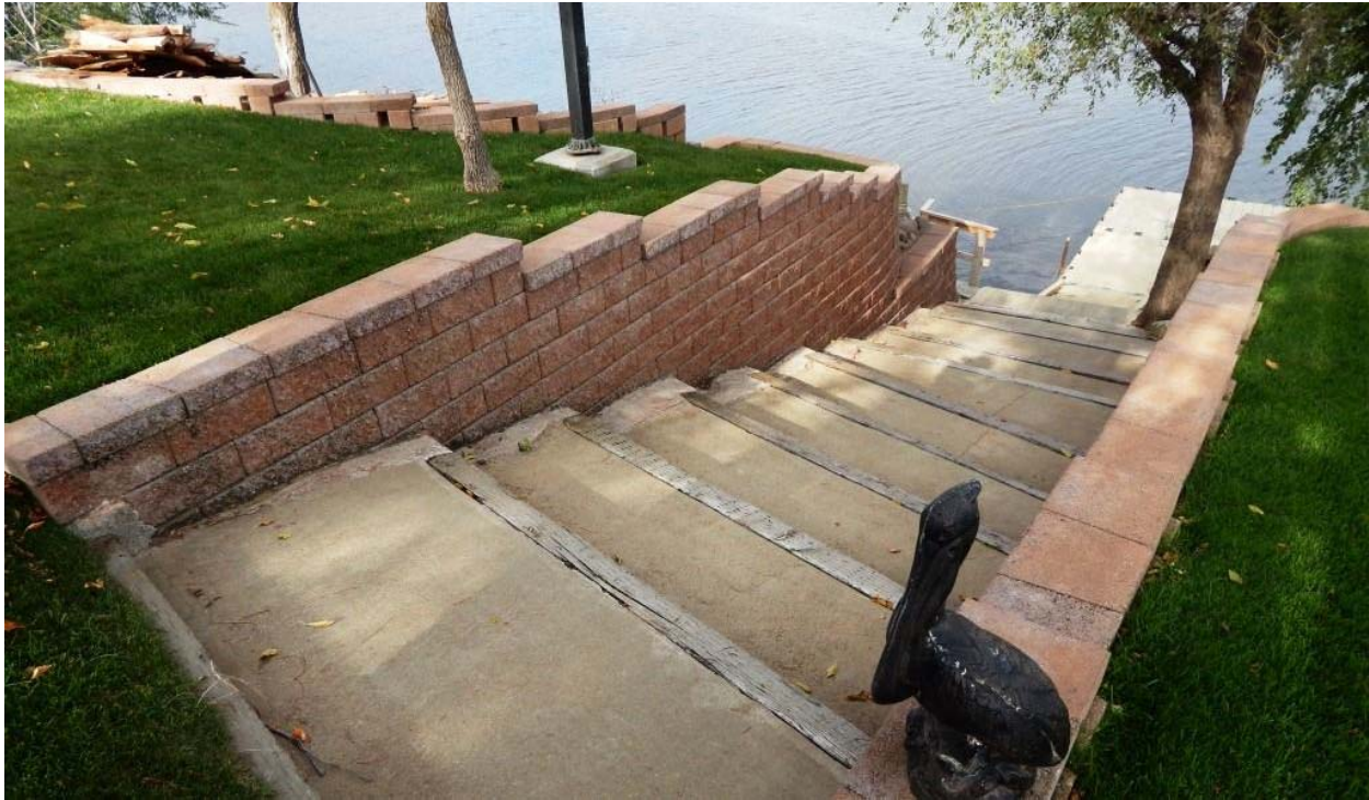
This picture was taken looking west. The steps that descend to the reservoir were constructed by the tenant of Cabin Site 3. There is also a floating dock in the right background. Many improvements to lake access have been constructed by various tenants throughout the reservoir's lake sites. Improvements, including docks, are allowable on the sites subject to approval by Reclamation and Dickinson's Parks and Recreation. (Bradshaw, 10-08-14)
