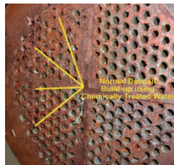
Figure 1. Low-Pressure Compressor 1 Heat Exchanger prior to water treatment demonstration (Courtesy of Flozone Services)
