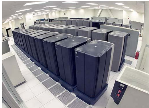
Figure 5-26. Typical Data Center
