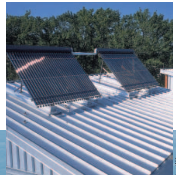
Smaller solar hot water systems, such as the system installed at the Chesapeake Bay Foundation's Philip Merrill Environmental Center in Annapolis, Maryland, are more common than larger systems, such as that found on the LANL Otowi Building.
