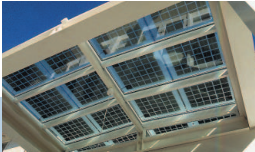
The skylighted entryway at the Thoreau Center for Sustainability at Presidio National Park, San Francisco, California, uses photovoltaic cells that are laminated to the skylight glass to produce electricity as well as to shade and daylight.
