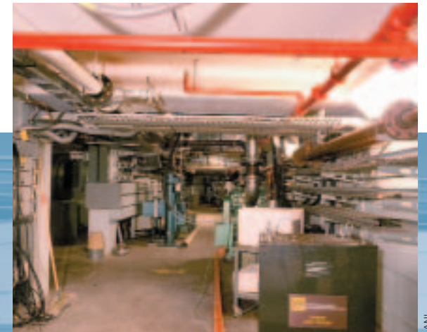
The LANL Ion Beam Facility mechanical room.
