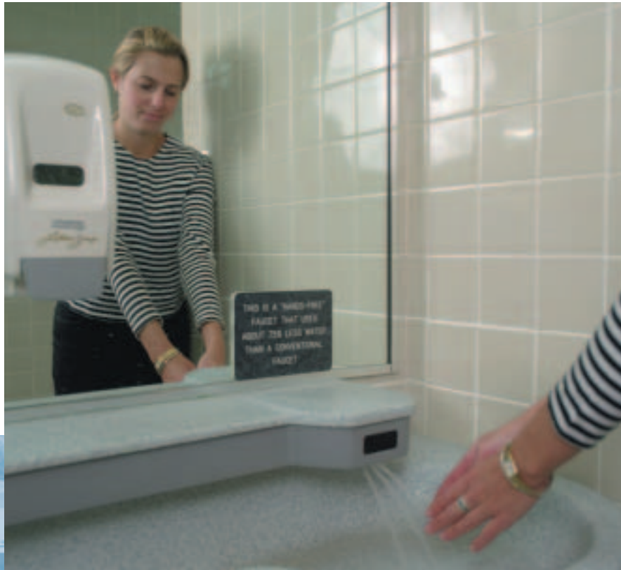
Sensors that automatically shut off faucets and flush toilets improve hygiene, comply with Americans with Disabilities Act (ADA) requirements, and save water.
