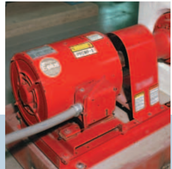
Perform functional tests at design, intermediate, and minimum flow conditions on variable frequency drive motors controlling variable flow hydronic systems.
