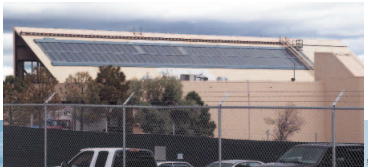
Solar hot water system on the LANL Otowi Building. The excellent solar resources in Los Alamos make solar hot water systems a viable solution for meeting DHW loads and preheating water for process and space heating loads. These systems have a high first cost, but very low operating costs. A year-round water heating load, such as for cafeteria, locker room facilities, and process loads, is required to make solar hot water systems cost-effective.
