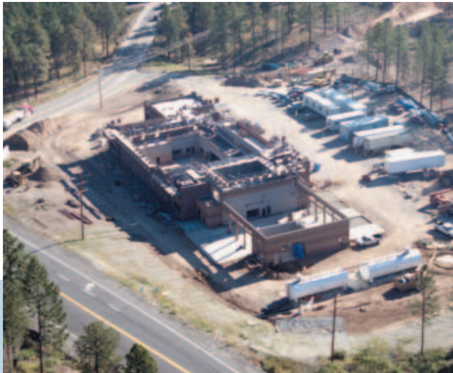
CMU construction for the LANL Emergency Operations Center provides a durable exterior wall. A second CMU interior wall provides mass to improve interior thermal comfort.
