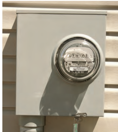
Meters measure a customer's use of electricity so that bills are accurate.
