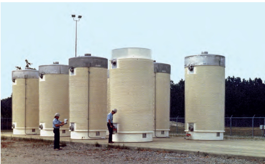
These dry storage casks hold spent nuclear fuel assemblies that have cooled for at least one year.
