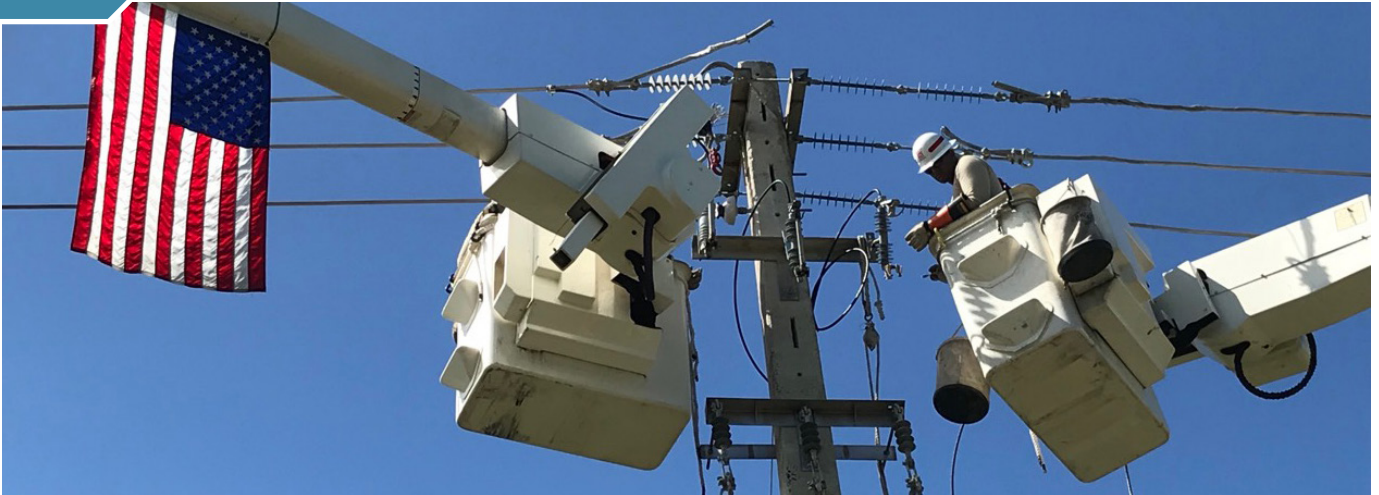
Linemen working to restore power in Puerto Rico after Hurricane Maria in 2017
